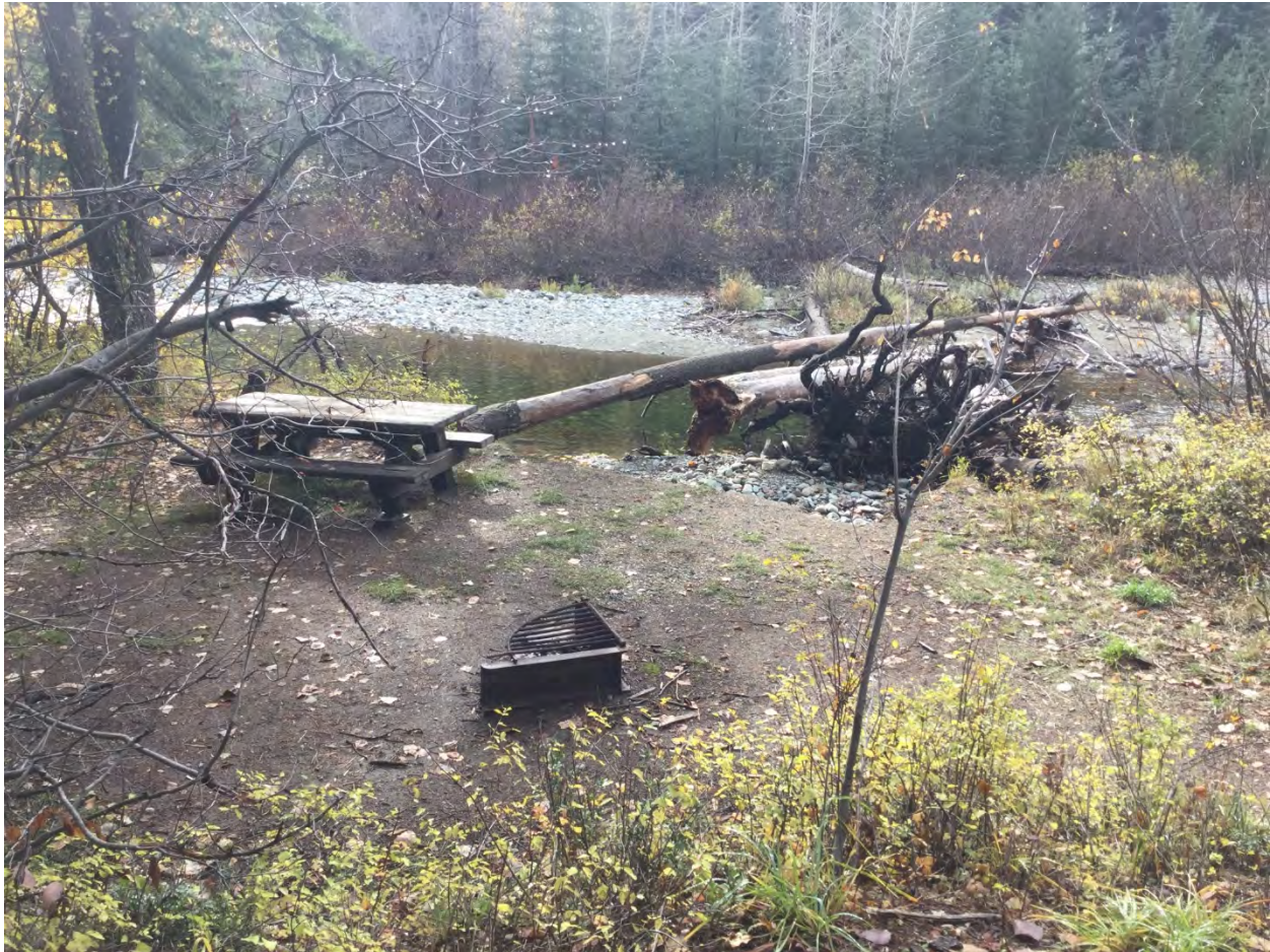
Figure 2-5. Photograph of Eroding Bank at the Poplar Flats Campground in the Upper Twisp River Reach 3 near RM 24.2
