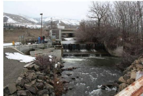
BEFORE: Bruton Dam blocks fish passage
