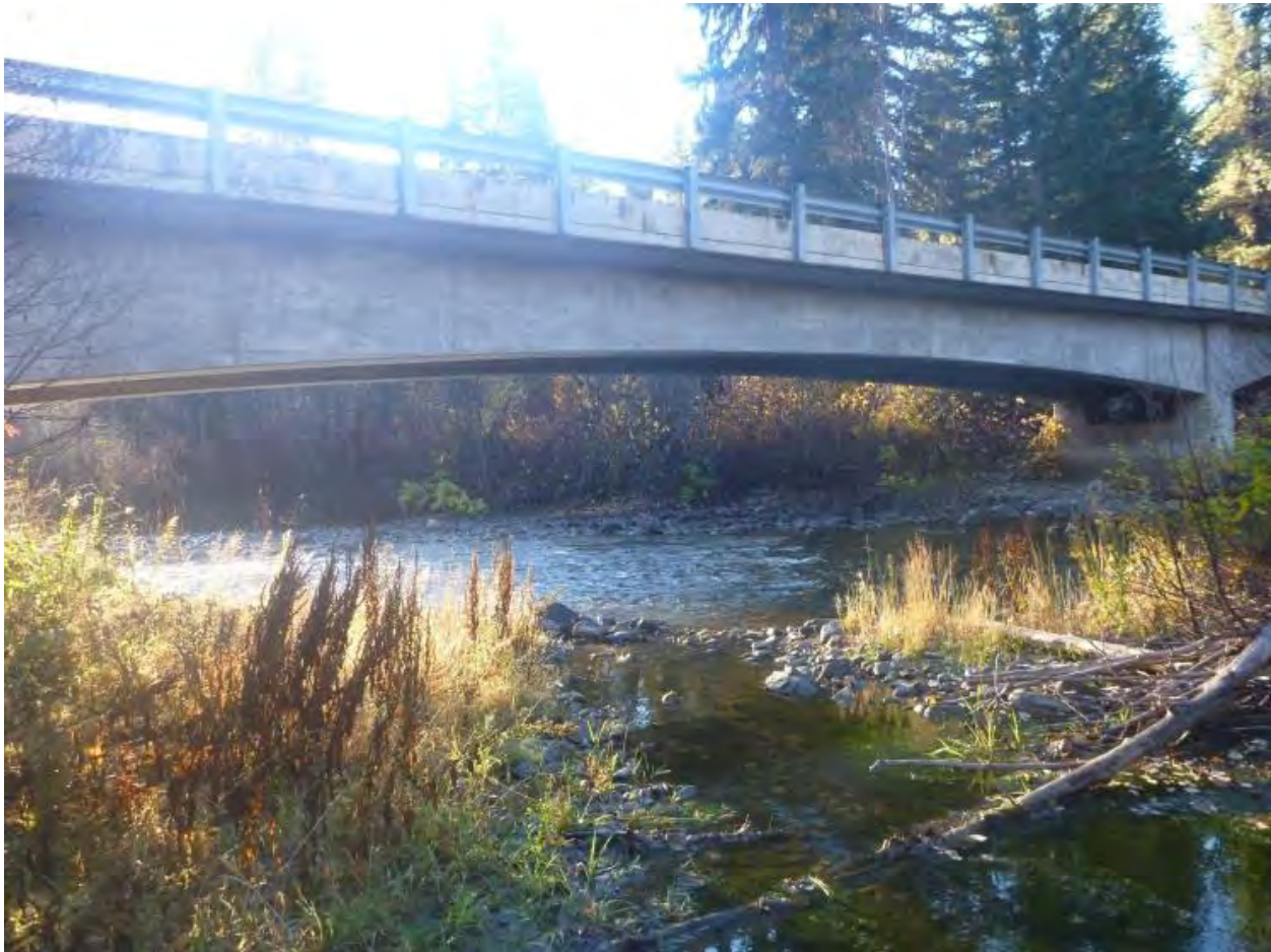
Figure 92. Channel spanning bridge at RM 18.12, the upstream extent of this geomorphic study.
