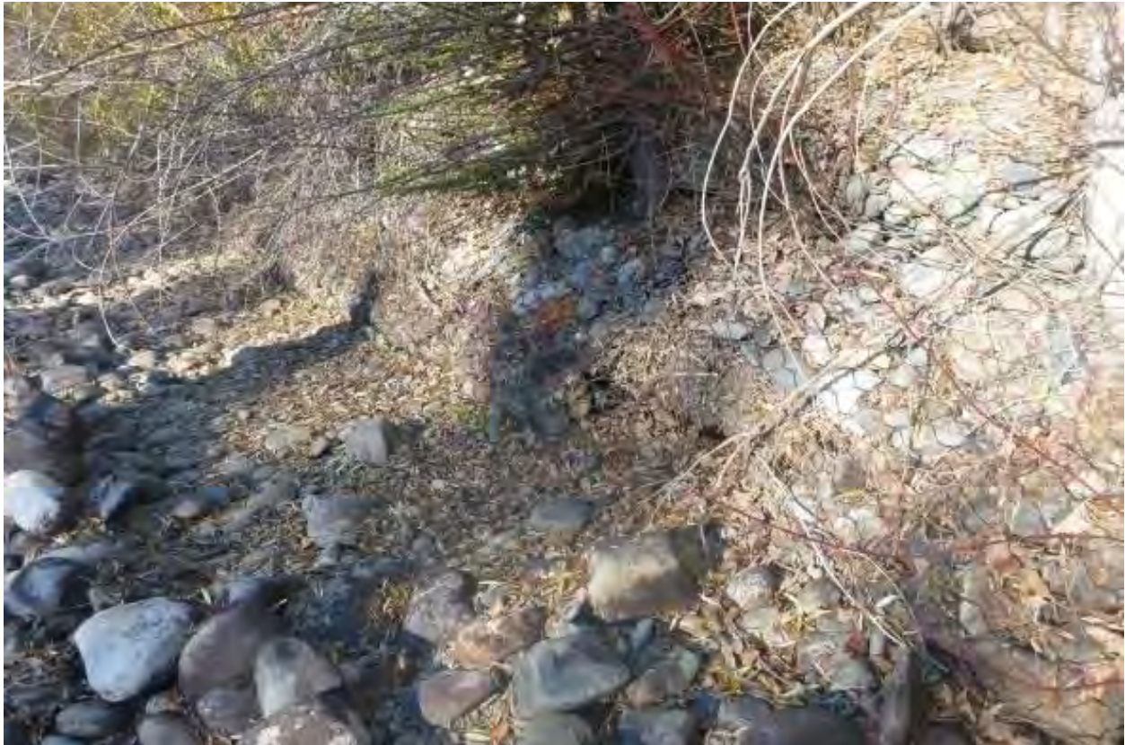
Figure 78. Gabion wall and culvert located at the upstream end of the large pond complex along river left at RM 16.1.
