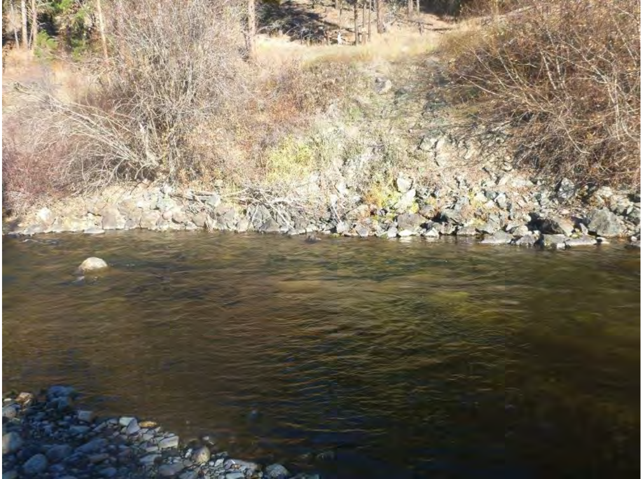
Figure 46. RM 10.27 river left, the road embankment and large angular riprap installed at the bank toe.
