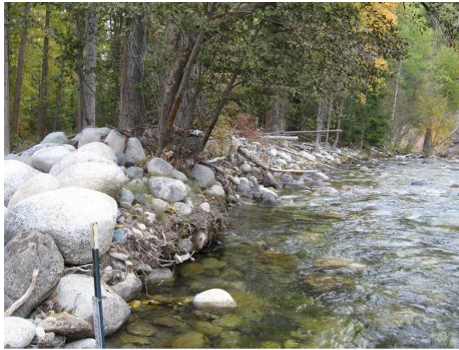
Figure 36. View to the southeast in the downstream direction at a push-up levee near RM 6.65 (October 2009).
