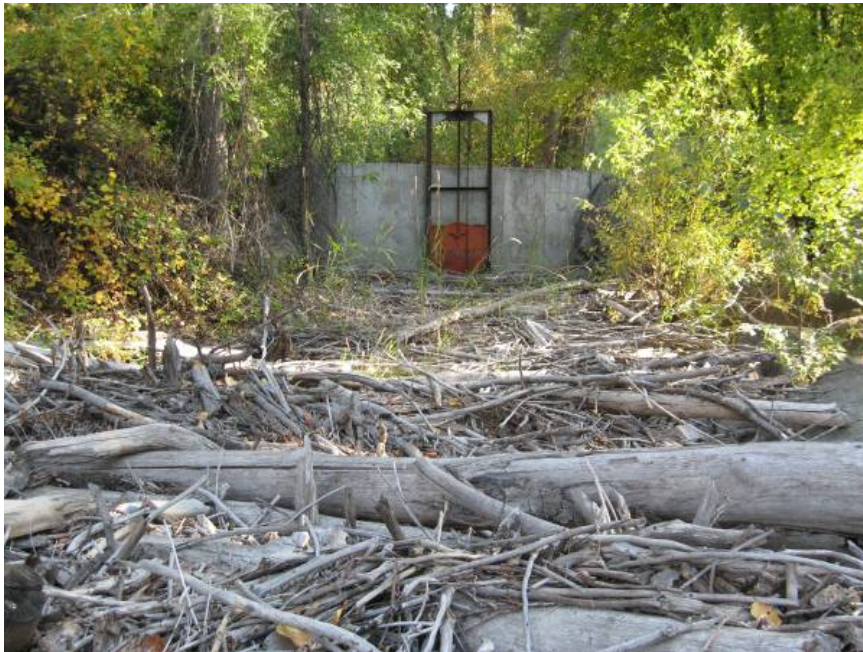
Figure 20. Headgate on river-left at RM 1.3 (October 2009).
