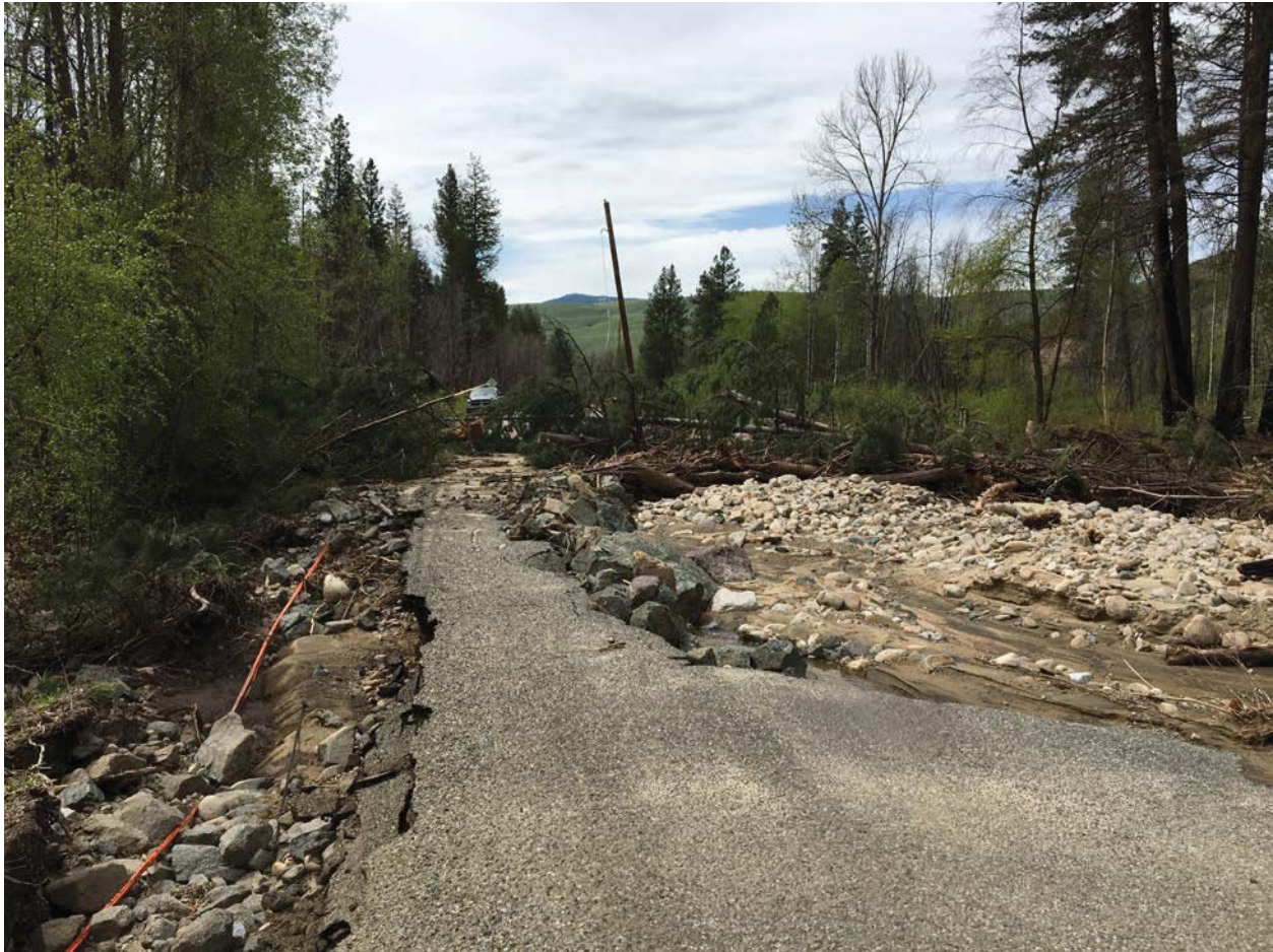
Figure 2-10. Photograph of Road Erosion in May 2017 (Source: J. Johnson)
