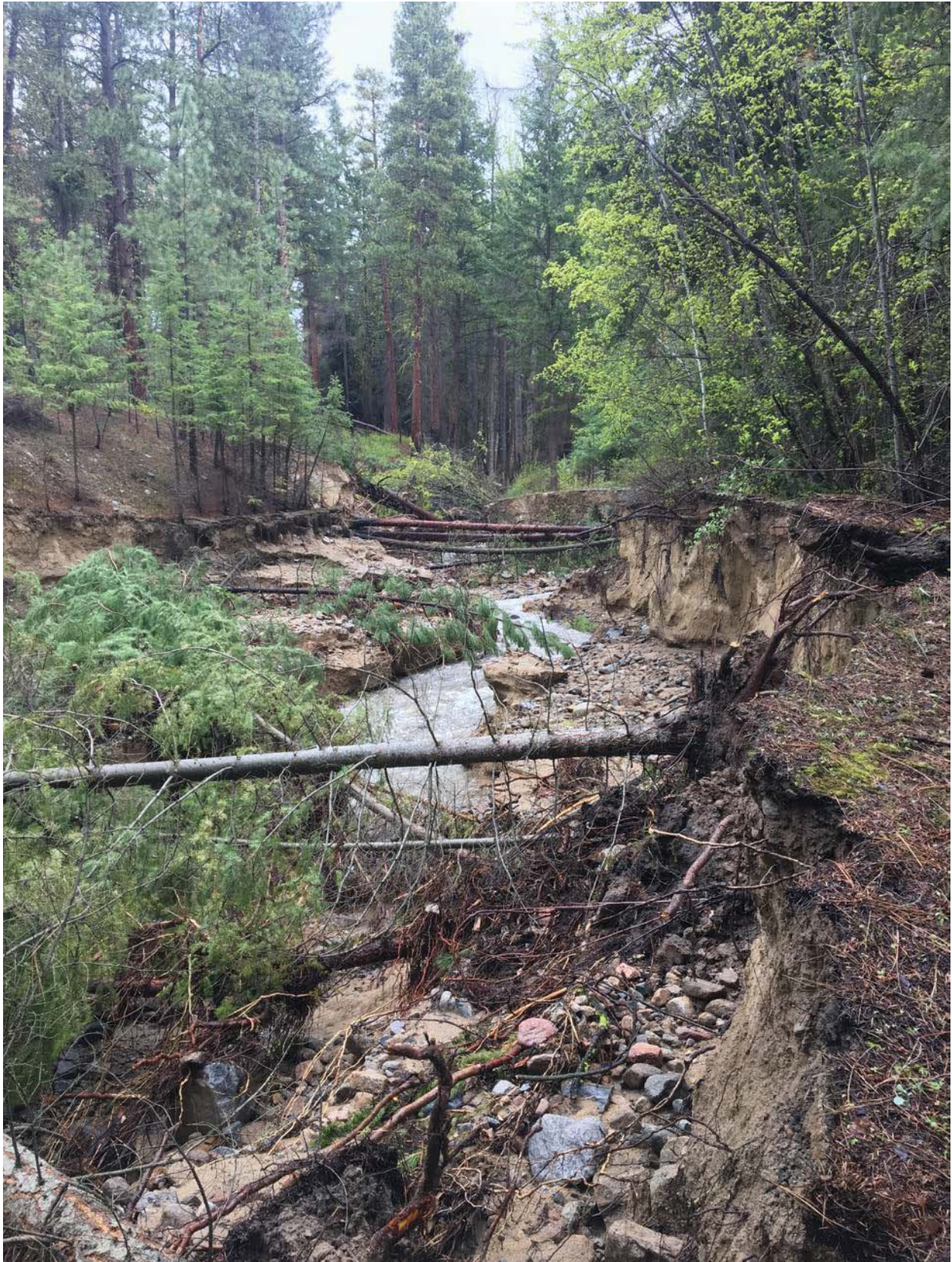
Figure 2-5. Photograph of Road Crossing Failure Location on Volstead Creek (Source: J. Johnson)
