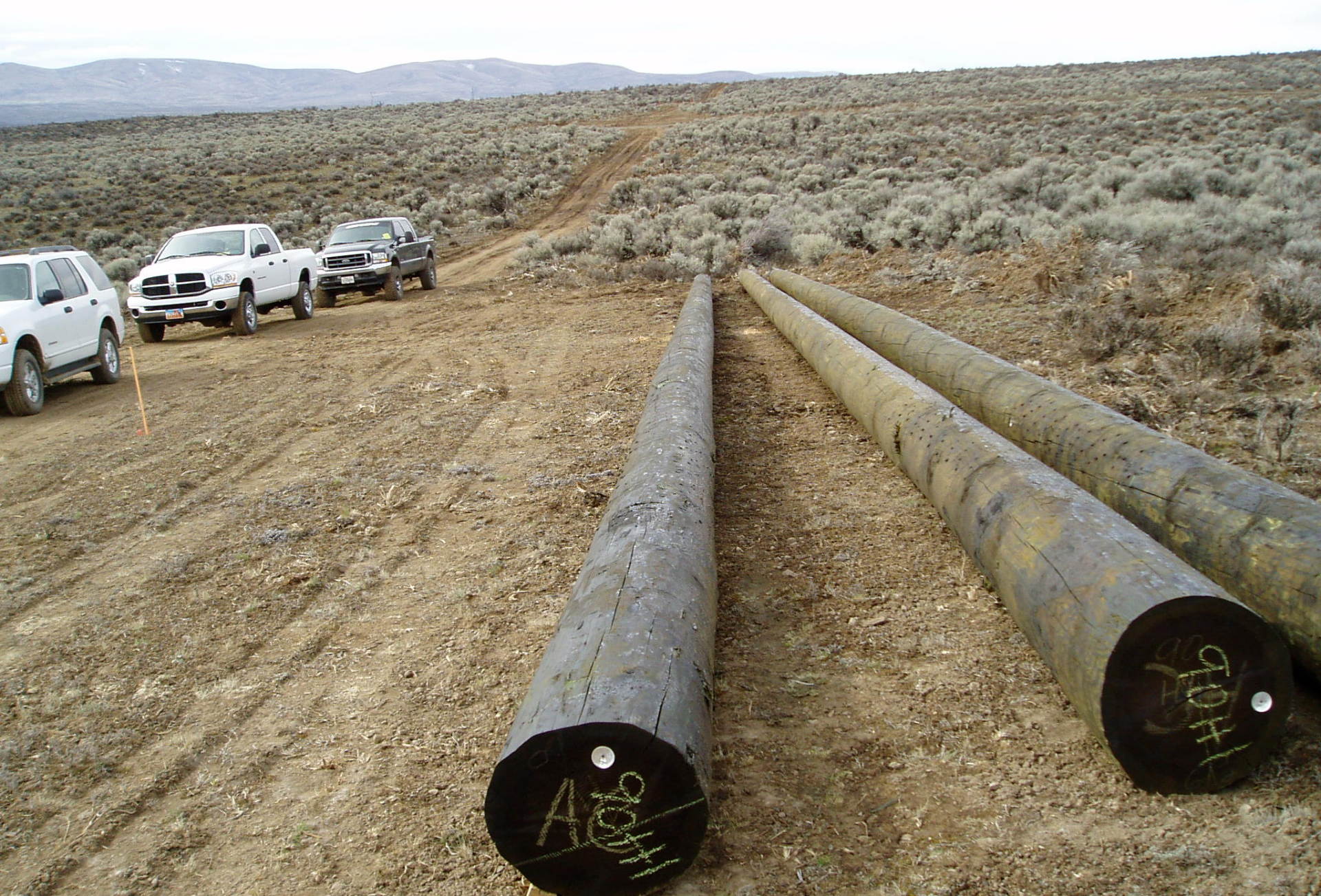
230 KV Overhead Feeder Line Pole Site
