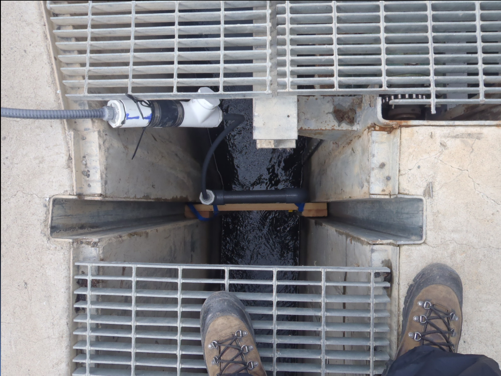
Primary Fish Bypass Pipe PIT tag antenna
