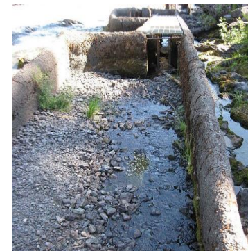
Non-functional Denil fish ladder at low flow
