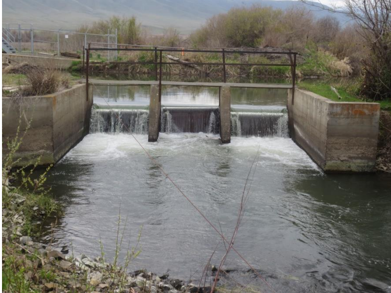
Figure 8. Unit 2 Diversion Dam in Toppenish Creek (river km 44.6), right channel looking downstream, a potential partial passage barrier for upstream migrating adult Pacific Lamprey.
