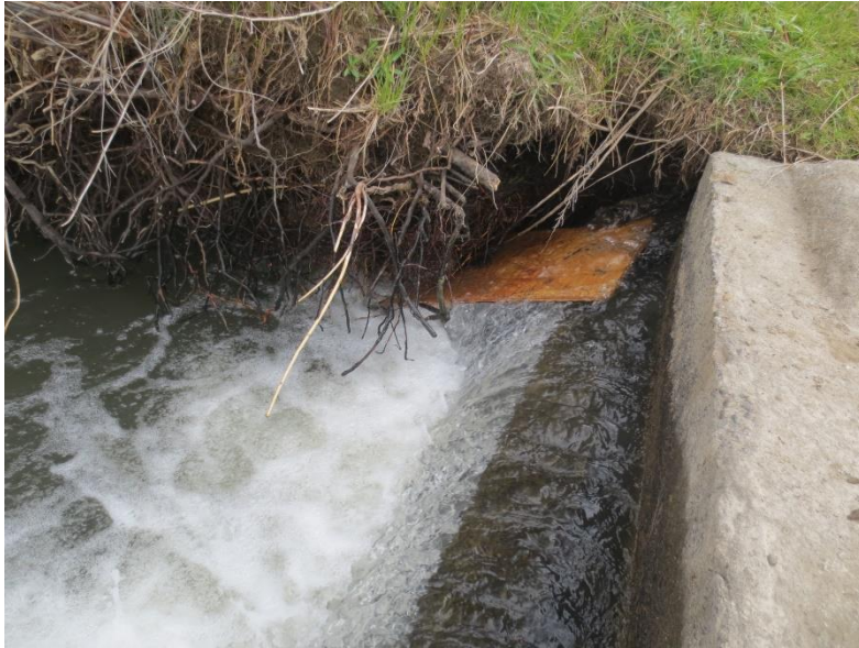
Figure 10. Plywood board inserted into the right bank of the left channel to improve adult Pacific Lamprey passage over Unit 2 Diversion Dam in Toppenish Creek (river km 44.6).
