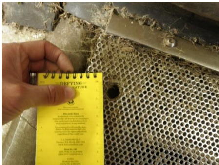
Figure G3-6. One of the four large openings (18 mm wide) on the first screen (perforated mesh 4.5 mm) of Chandler Diversion Juvenile Monitoring Facility.
