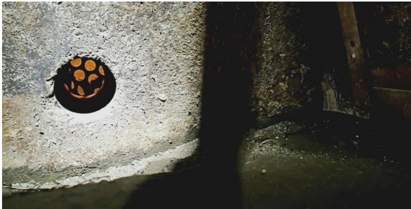
Figure G5-6. Exterior view of the lamprey exit hole in the Roza fish facility holding tank during the fall maintenance drawn down of the forebay. The perforated plate visible through the hole is part of the fish crowder.
