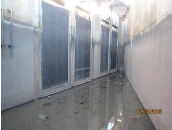
Figure G3-2. Location where the three bypass routes converge (looking downstream) - traveling belt screens on the left protecting the pump stations (two bays, four screens).
