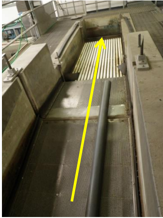
Figure G3-5. First segment of CJFMF looking downstream (yellow arrow shows direction of water and fish). Perforated screen is ~20 ft long (upslope), bar screen is ~4 ft (downslope), and the PVC section is ~10 ft long.
