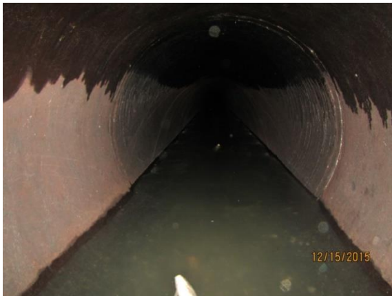
Figure G3-4. Concrete conduit leading to Chandler Diversion Juvenile Monitoring Facility (looking inside). This entire route was not examined.
