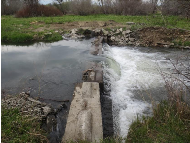
Figure E1-2. Unit 2 Diversion Dam in Toppenish Creek (river km 44.6), left bank looking downstream, a potential partial passage barrier for upstream migrating adult Pacific Lamprey.
