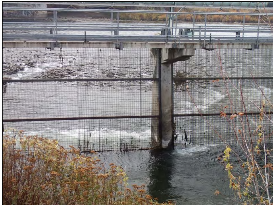
Figure 21. The Roza Wasteway #2 outfall screen structure at the Yakima River confluence, with the gravel bar visible beyond screen.
