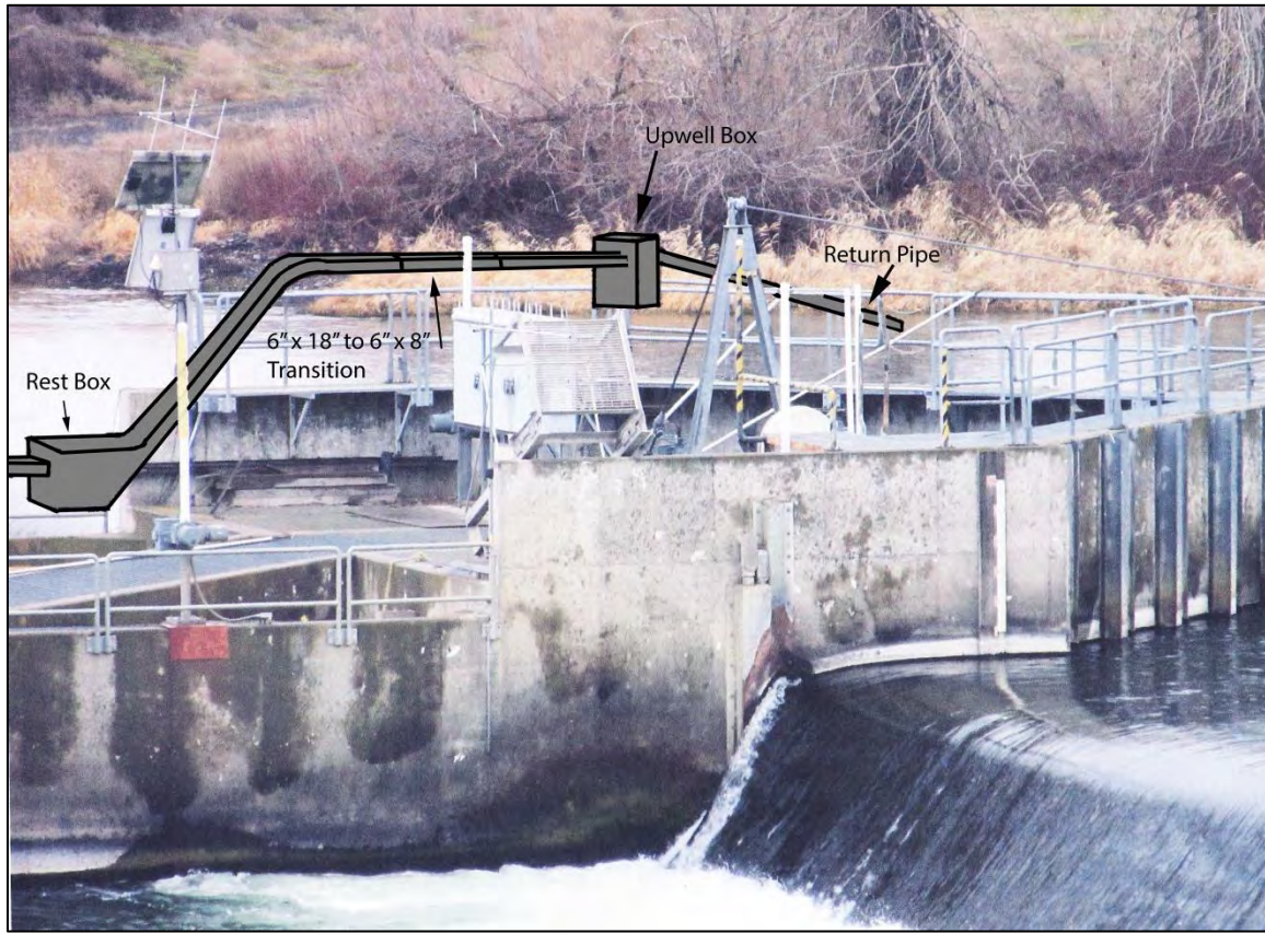
Figure 26. Photograph of center fishway at Sunnyside Dam with concept drawing of LPS that returns lamprey to river upstream of dam instead of into fish ladder as shown in Figure 25 (J. Simonson, Fishhead Technology).
