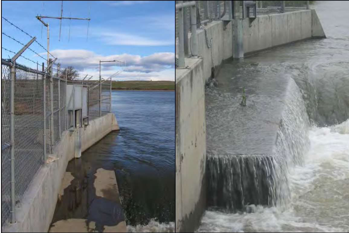
Figure 15. The ledge on the right bank of Wanawish Dam that it appears most Pacific lampreys used to pass upstream. The flow is approximately 5,500 ft 3 /s in the left picture and 10,500 ft 3 /s on the right. The entrance to the fishway is just out of the picture on the left hand side.
