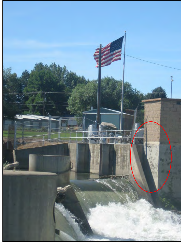
Figure A-3. Prosser dam and the head of the Chandler Canal. The ramp would be placed in the space (circled in red) between the gate house and the slanted wall at the left bank of the dam.
