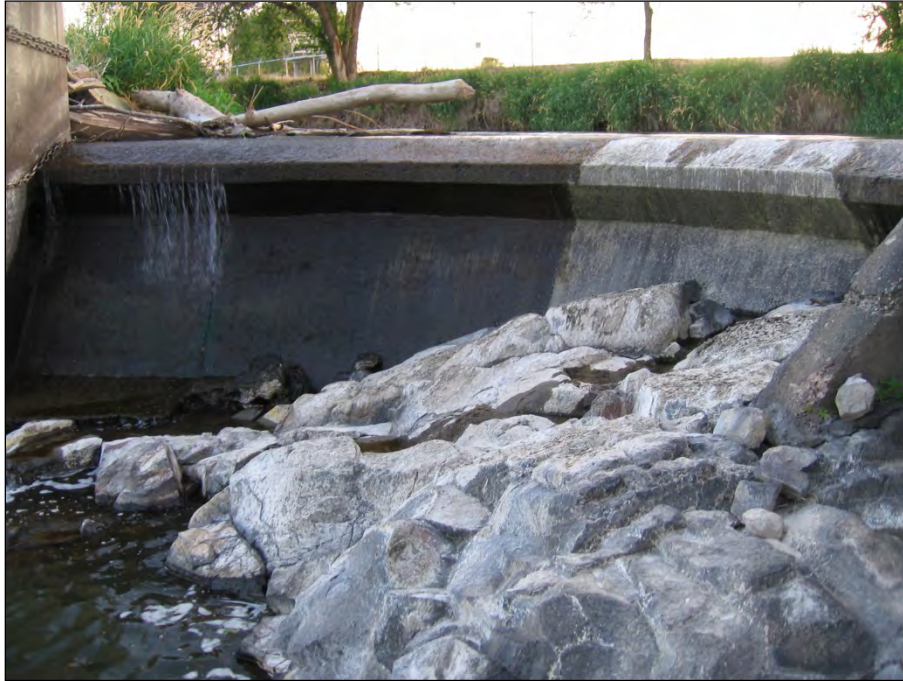
Figure A-7. Proposed site at Prosser Dam of rock ladder showing bedrock at low flow. The head of the Chandler Canal is just right of the edge of the frame.
