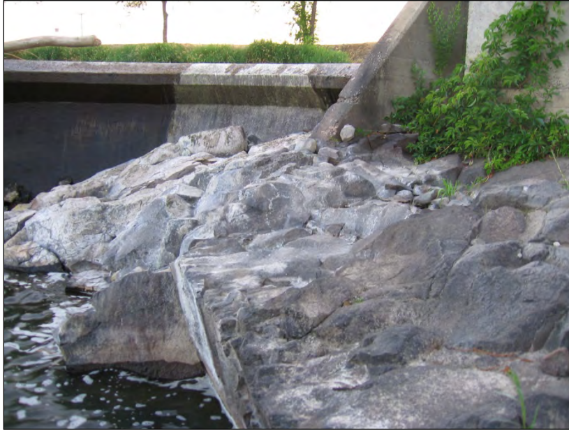
Figure A-2. Proposed site of LPS on the left bank of Prosser Dam at low flow.
