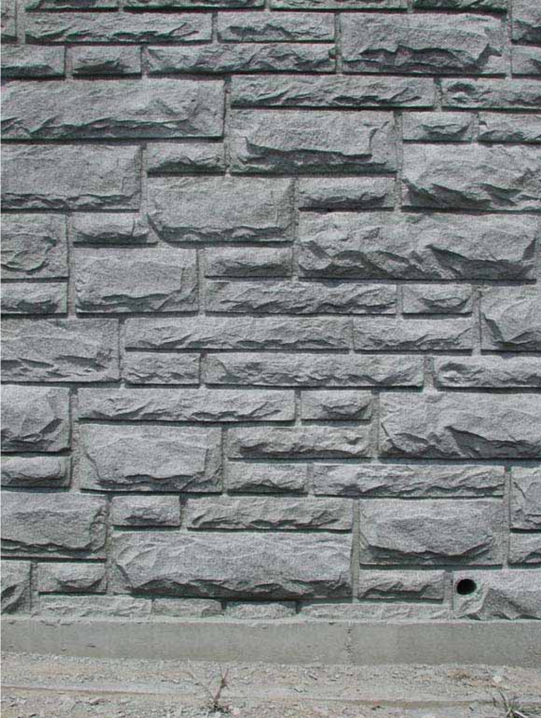
Figure 5 – This concrete retaining wall on the Blue Ridge Parkway bears a split-face granite texture and color produced with the use of form liners and concrete stain. The pattern is a three-height, random ashlar, and was custom made to give the same appearance as the natural stone retaining walls of the Parkway.
