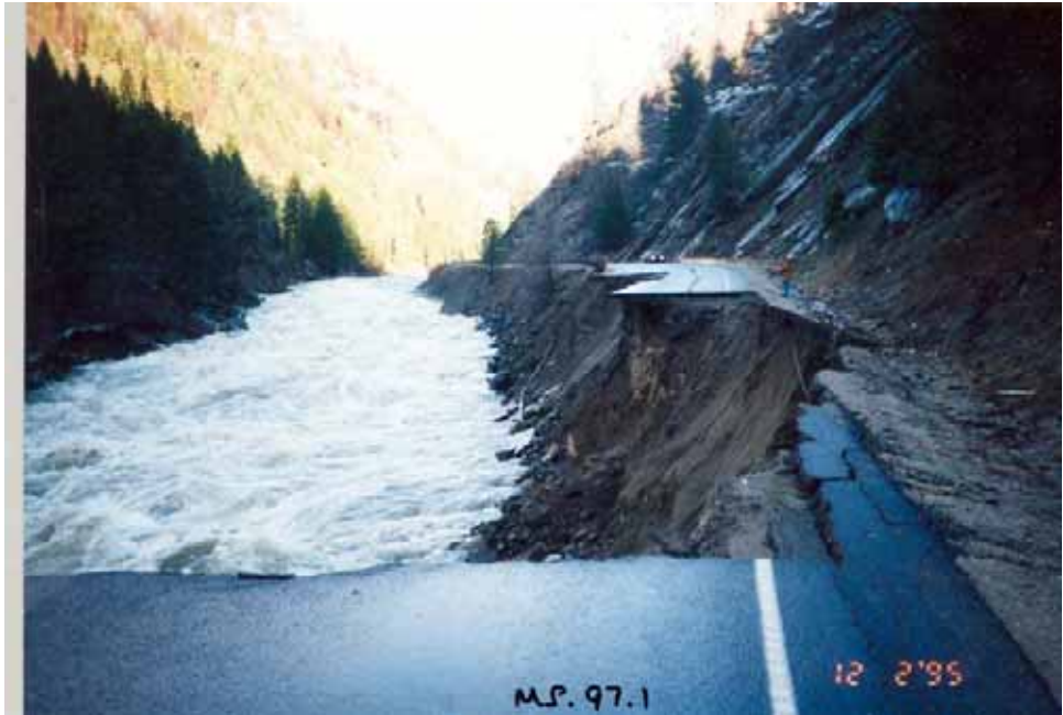
Figure 1 - Failure occurring at Mile Post 97.1, Washington US-2, on December 2, 1995. One can envision a roadway prism moved upslope, away from the Wenatchee River, supported by retaining walls and other structure, as seen in the figure below.
