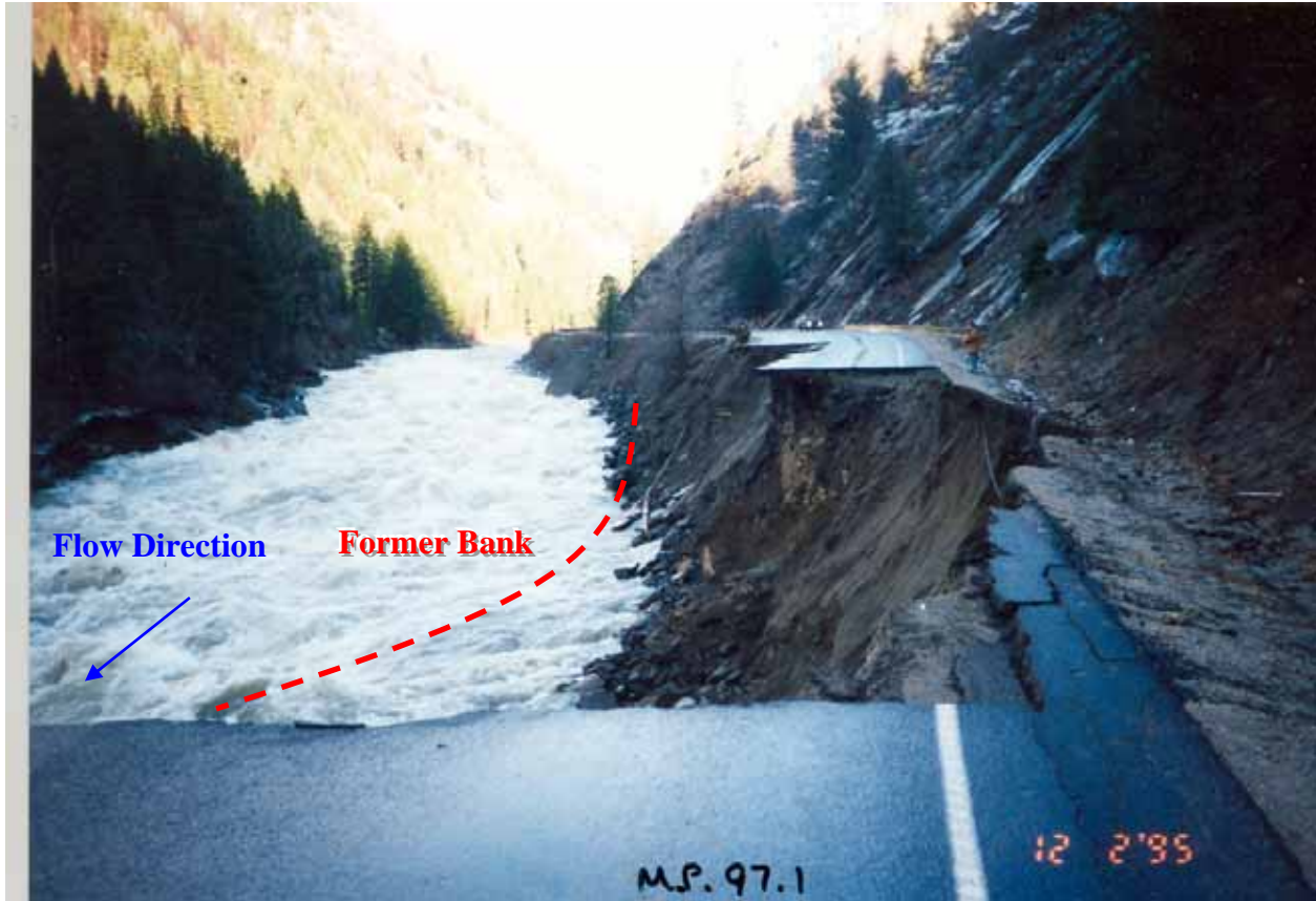
Figure 2-3. Road Washout at MP 97.10 on November 30, 1995.
