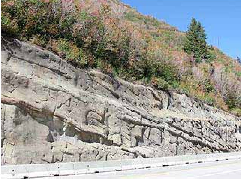
Figure 6 - This concrete facing seen on U tah 189 through Provo Canyon, is designed and built to cover the soil and rock stabilization beneath, and to m im ic the native stone in bedding plane, color and texture. The slope stabilization system included a combination of soil nails and rock dow els covered by a temporary shotcrete facing (soil nails only) and a cast-in-place form ed finish concrete facing covering all the treated areas.
