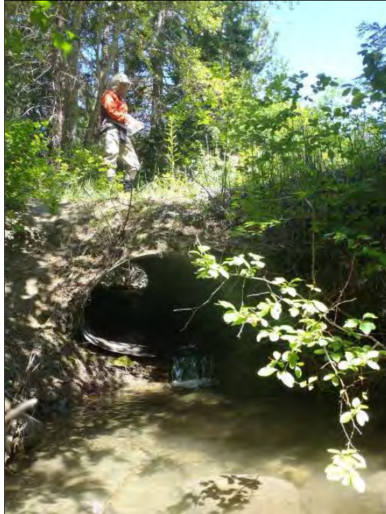
Figure 45. Perched culvert in Deadhorse Creek (RM 38.6). Surface water connection was present on day of survey (July 26, 2011).
