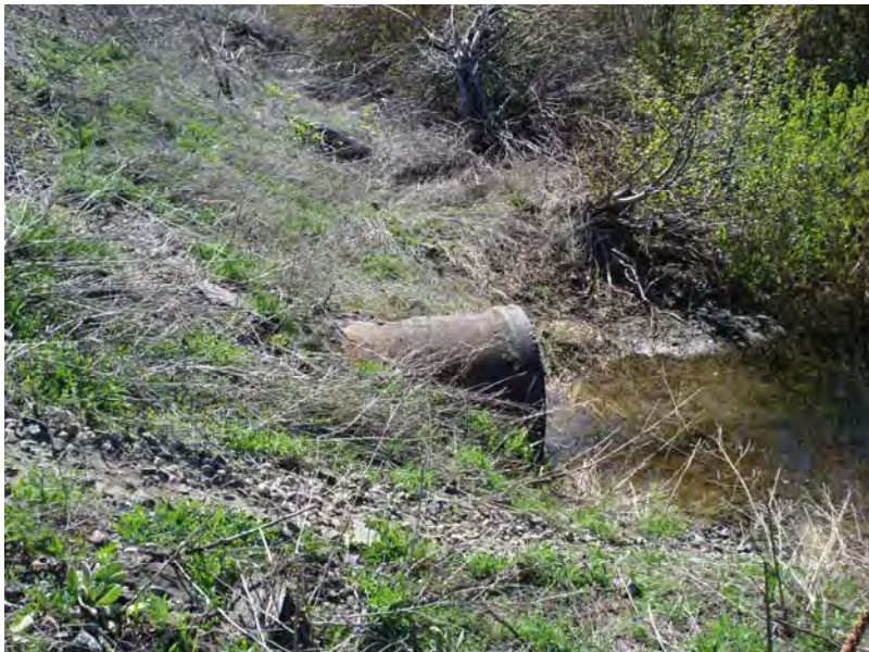
Figure 25 - Culvert that drains the wetlands on the south side of the railroad grade at the downstream end of the subreach, view to the southeast. Lower White Pine Reach; Subreach DIZ-1, Nason Creek - Wenatchee Subbasin, Washington. Bureau of Reclamation Photograph by R. McAfee, May 5, 2007.
