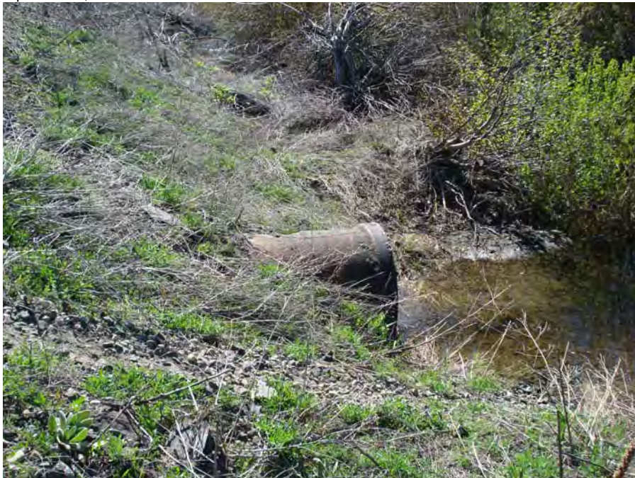
Photograph No. 5. View to the southeast of the culvert that drains the wetlands on the south side of the railroad grade at the downstream of the subreach. Lower White Pine Reach; Subreach DIZ-6, Nason Creek - Wenatchee Subbasin, Washington. Bureau of Reclamation Photograph by R. McAfee, May 5, 2007.
