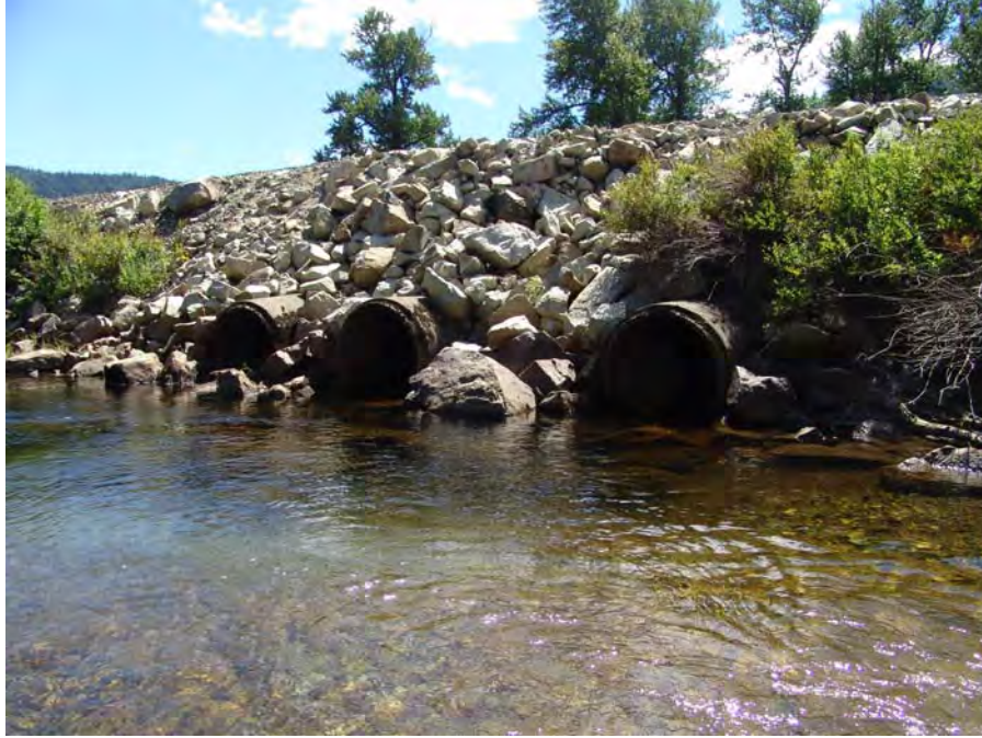
Photograph No. 14. View is to the south looking at three concrete culverts that run through the railroad grade on the right bank. The culverts drain the area of LWP DIZ-2 and LWP DOZ-4. Lower White Pine Reach; Subreach IZ-5, Nason Creek - Wenatchee Subbasin, Washington. Bureau of Reclamation Photograph by D. Bennett; August 8, 2007.
