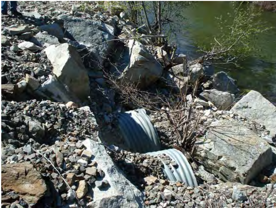
Photograph No. 13. View to the northwest of three elevated metal culverts that run through the railroad grade and drain the area of LWP DIZ-2 and LWP DOZ-4. Lower White Pine Reach; Subreach IZ-5, Nason Creek - Wenatchee Subbasin, Washington. Bureau of Reclamation Photograph by R. McAfee; May 4, 2007.
