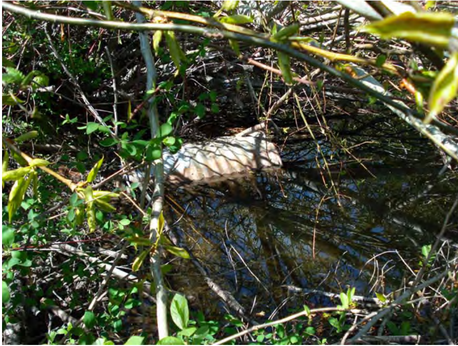
Photograph No. 4. View of the culvert that drains the wetlands on the north side of Highway 2. Lower White Pine Reach; Subreach DOZ-8a, Nason Creek - Wenatchee Subbasin, Washington. Bureau of Reclamation Photograph by R. McAfee, May 3, 2007.
