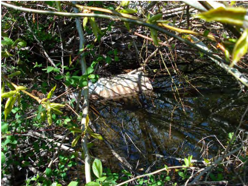
Figure 28 - Culvert that drains the wetlands on the north side of Highway 2. Lower White Pine Reach; Subreach DOZ-3, Nason Creek - Wenatchee Subbasin, Washington. Bureau of Reclamation Photograph by R. McAfee, May 3, 2007.
