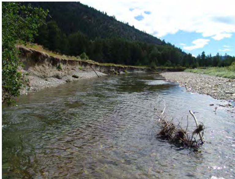
Figure 36 - Accelerated erosion along the cleared left bank, view is to the east looking downstream. Lower White Pine Reach; Subreach IZ-2, Nason Creek - Wenatchee Subbasin, Washington. Bureau of Reclamation Photograph by D. Bennett; August 8, 2007.
