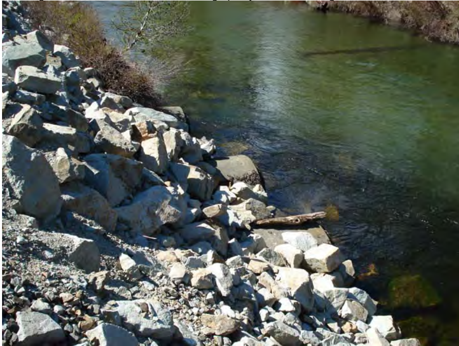
Photograph No. 15. View to the northwest of three concrete culverts that drain the area of LWP DIZ-2 and LWP DOZ-4. Lower White Pine Reach; Subreach IZ-5, Nason Creek - Wenatchee Subbasin, Washington. Bureau of Reclamation Photograph by R. McAfee; May 4, 2007.
