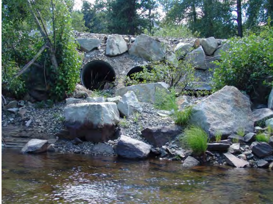
Photograph No. 12. View is to the south of elevated corrugated through the railroad grade that acts as the right bank. The culverts drain the area of LWP DIZ-2 and LWP DOZ-4. Lower White Pine Reach; Subreach IZ-5, Nason Creek - Wenatchee Subbasin, Washington. Bureau of Reclamation Photograph by D. Bennett; August 8, 2007.
