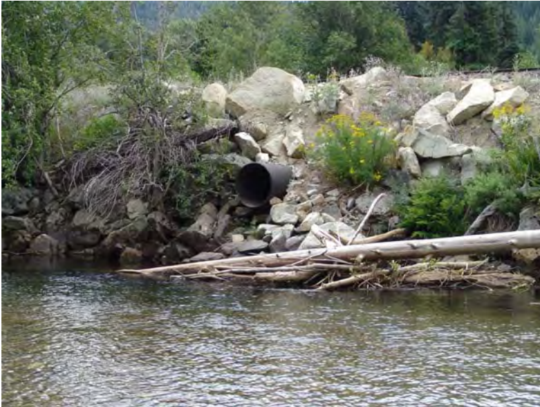
Figure 52 - Elevated culvert through the railroad grade that drains run off water from the area of LWP DIZ-1 and LWP DOZ-2, view is to the south. Lower White Pine Reach; Subreach IZ-3, Nason Creek - Wenatchee Subbasin, Washington. Bureau of Reclamation Photograph by D. Bennett; August 8, 2007.
