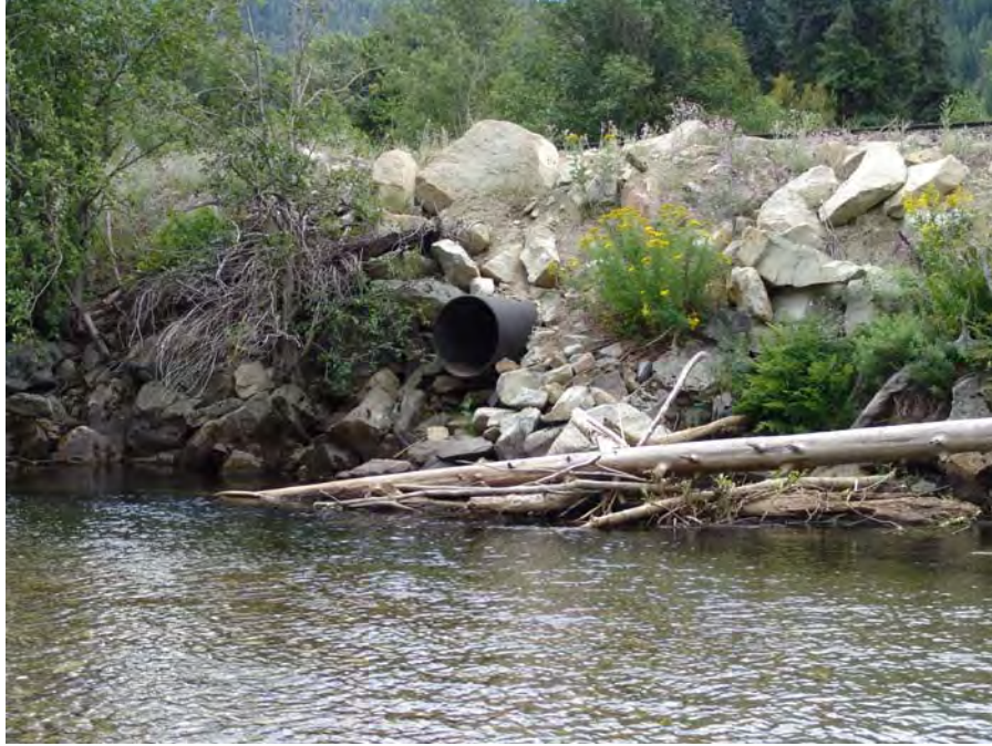
Photograph No. 10. View is to the south looking at an elevated culvert through the railroad grade that drains run off water from the area of LWP DIZ-2 and LWP DOZ-4. Lower White Pine Reach; Subreach IZ-3, Nason Creek - Wenatchee Subbasin, Washington. Bureau of Reclamation Photograph by D. Bennett; August 8, 2007.
