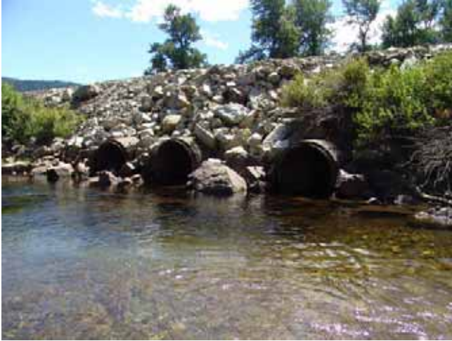
Figure 7. View to the south near RM 9.7 looking at the right river bank with concrete culvert inverts at water surface level. (Reclamation photograph by D. Bennett, August 8, 2007).
