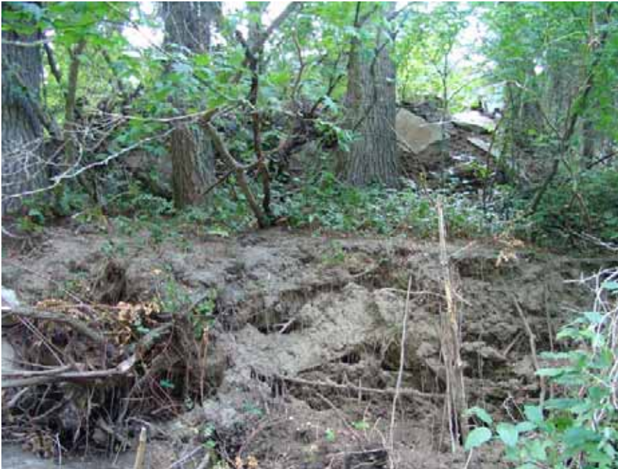
Figure 24. View is to the south looking at the right bank showing original ground level with fill material on top at river bank adjacent to Merritt. (Reclamation photograph by D. Bennett, August 8, 2007).
