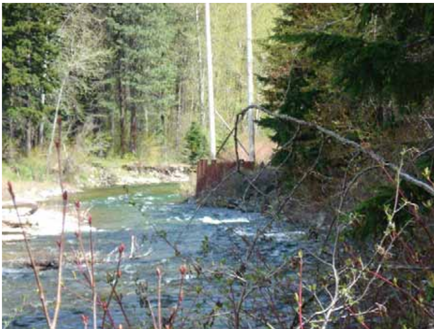
Figure 30. Downstream view to the east of sheet pilings that protect the power pole near RM 13.5
