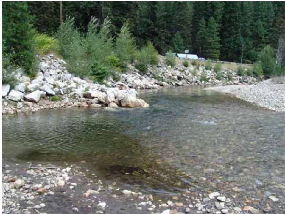
Figure 32. View is to the northeast looking downstream, showing riprap with two rock spurs into channel at RM 13.3. (Reclamation photograph by D. Bennett, August 7, 2007).
