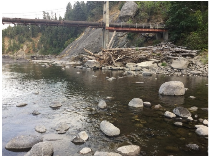
Figure 4-13. Photograph of Rare Log Jam Racked on a Crossing Abutment in Reach 8, near RM 22.8
