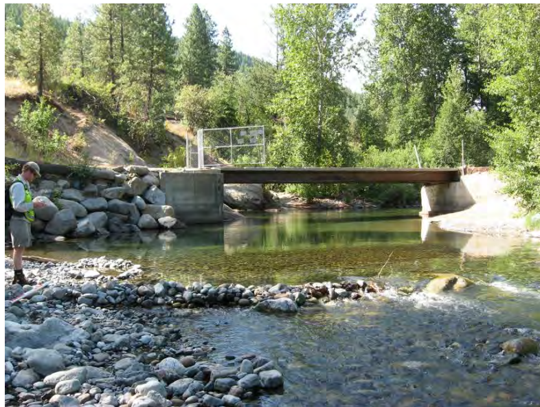
Figure 78. View looking toward the southwest in the upstream direction near river mile 6.45. This narrow private bridge creates hydraulic and geomorphic constraints on the channel and floodplain. Photo taken in August 2009.
