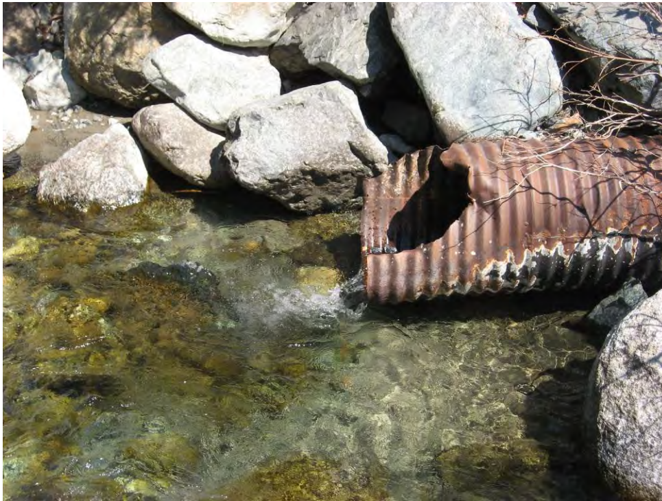
Figure 58. Culvert entering the mainstem on the river right bank near river mile 8.4.
