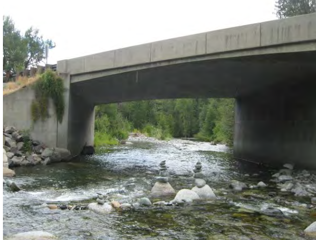
Figure 70. View toward the northeast in the downstream direction near river mile 5.0. The bridge at this location limits local channel dynamics, and floodplain connection downstream. Photo taken in August, 2009.
