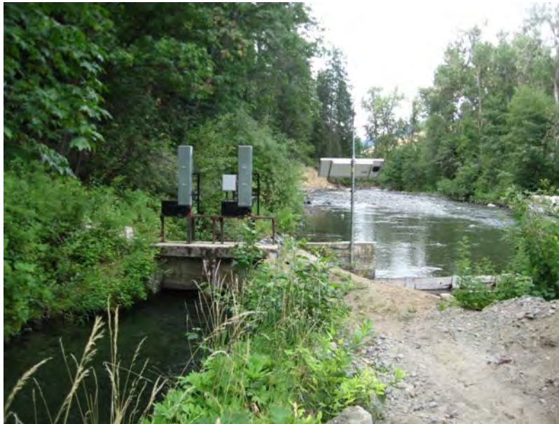
Figure 21. View looking upstream toward the southwest at the Peshastin Canal diversion near river mile 2.5.
