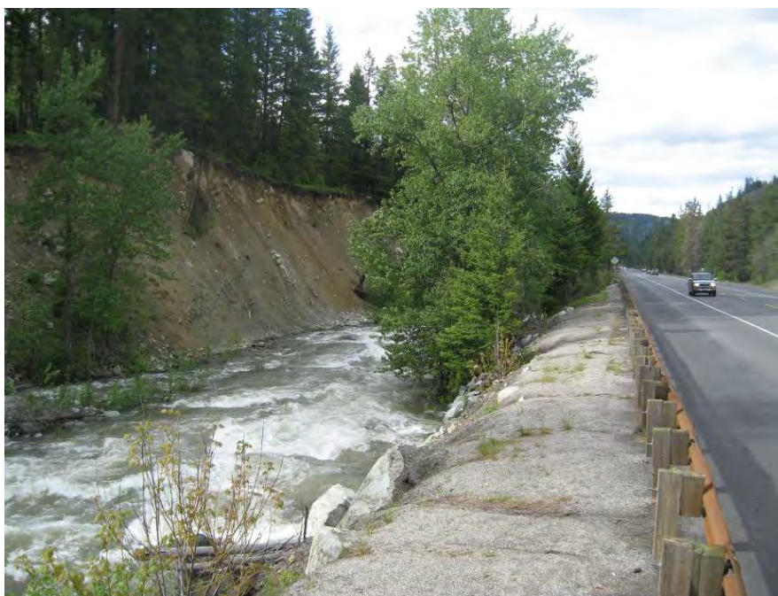
Figure 86. View downstream just downstream of the Ingalls Cr confluence. Hwy 97 directly abuts the channel and contributes to erosion of the high glacial terrace on the opposite bank (May 2010 Photo).
