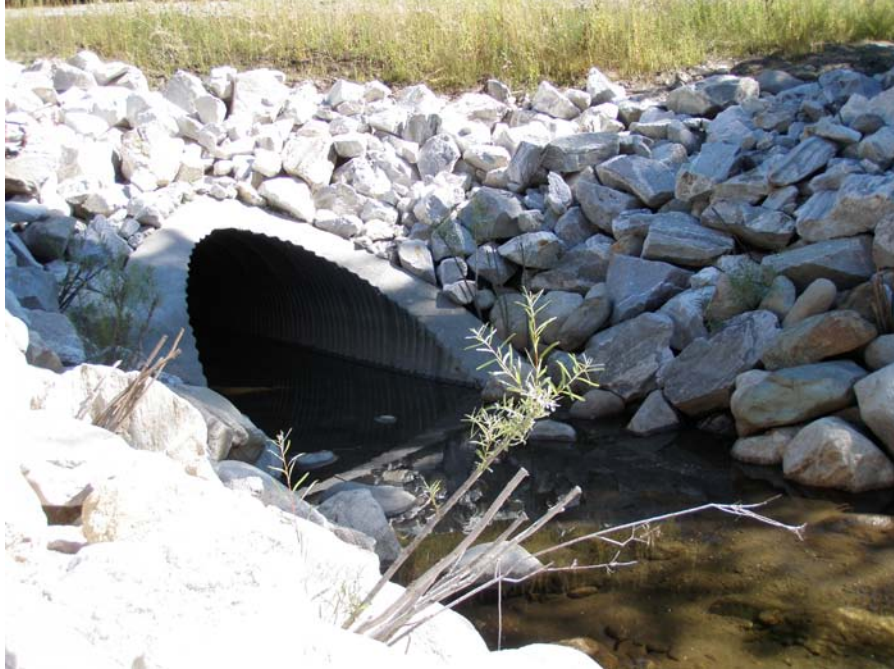
Photograph No. 15. View to the east looking downstream at culvert placed through improved road embankment that reconnects side channel. Lower Nason Creek, Wenatchee Subbasin, Washington – Bureau of Reclamation Photograph by E. Lyon, September 13, 2010.
