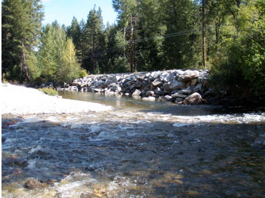
Photograph No. 7. View to the east looking downstream at riprap placed along river right protecting improved road. There is also a disconnected historic channel path behind the embankment. Lower Nason Creek, Wenatchee Subbasin, Washington – Bureau of Reclamation Photograph by E. Lyon, September 13, 2010.
