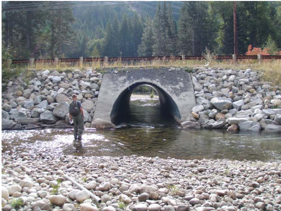
Photograph No. 42. View to the east looking at culvert through improved road embankment that reconnects historic channel path. Lower Nason Creek, Wenatchee Subbasin, Washington – Bureau of Reclamation Photograph by E. Lyon, September 15, 2010.
