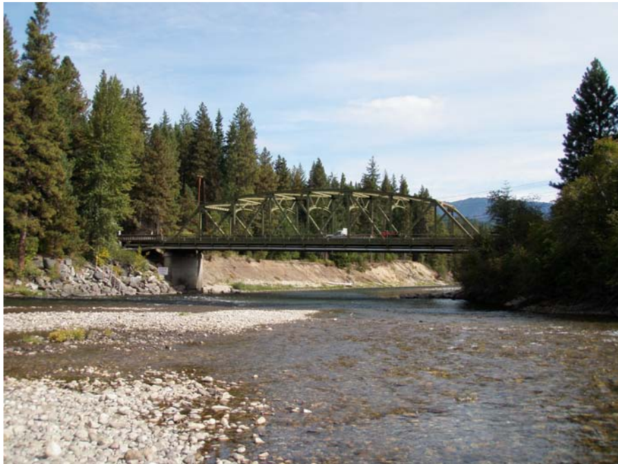
Photograph No. 54. View to the northeast looking at bridge crossing over the Wenatchee River downstream of the confluence with Nason Creek. Lower Nason Creek, Wenatchee Subbasin, Washington – Bureau of Reclamation Photograph by E. Lyon, September 16, 2010.
