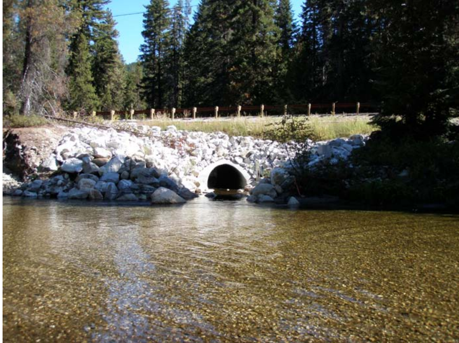
Photograph No. 33. View to the east looking at a culvert that reconnects a historic channel path that was blocked by an improved road. Lower Nason Creek, Wenatchee Subbasin, Washington – Bureau of Reclamation Photograph by E. Lyon, September 14, 2010.
