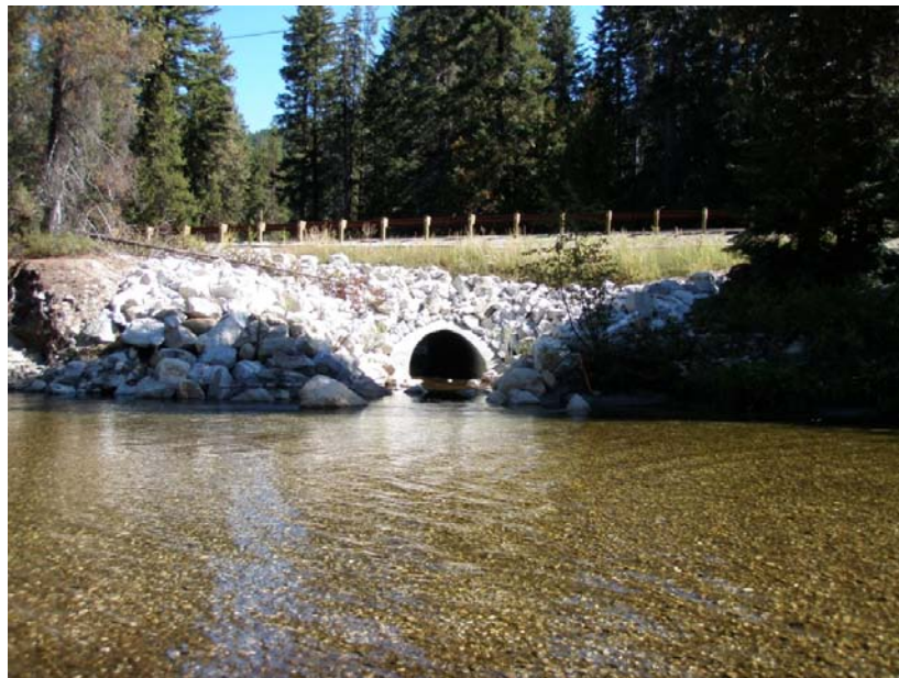
Figure 34. Channel Segment C: View looking at a culvert placed through the embankment of State Route 207 that reconnects a historic channel path (SC_1.17_R) near RM 1.30. Lower Nason Creek, Wenatchee Subbasin, Washington – Bureau of Reclamation Photograph by E. Lyon, September 14, 2010.
