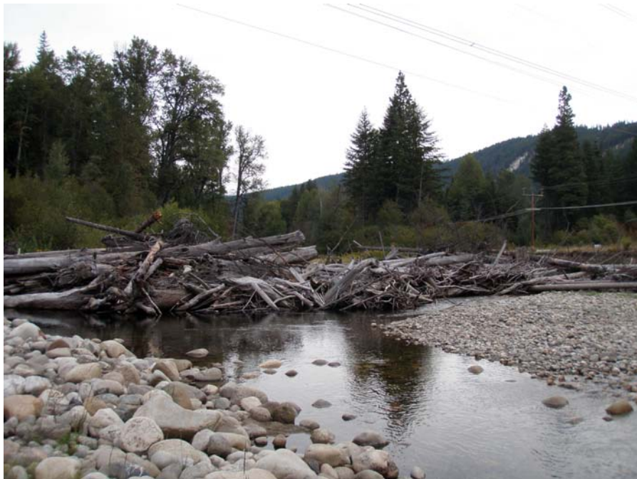
Photograph No. 36. View to the northeast looking downstream at large wood complex at head of side channel that may be contributing to bank erosion along river right. Lower Nason Creek, Wenatchee Subbasin, Washington – Bureau of Reclamation Photograph by E. Lyon, September 15, 2010.
