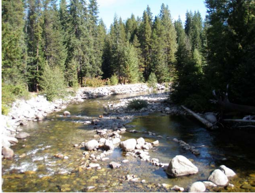
Figure 38. Channel Segment D: View looking from Nason Creek Campground Road bridge at riprap protecting campground along river left near RM 0.80. Lower Nason Creek, Wenatchee Subbasin, Washington – Bureau of Reclamation Photograph by E. Lyon, September 13, 2010.
