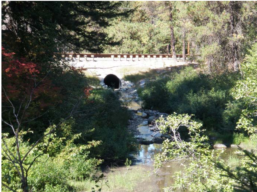
Photograph No. 12. View to the northwest looking downstream at a reconnected side channel through an improved road embankment along river right. Lower Nason Creek, Wenatchee Subbasin, Washington – Bureau of Reclamation Photograph by E. Lyon, September 13, 2010.
