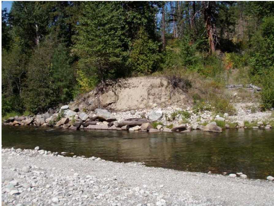
Photograph No. 58. View to the northwest looking at historic bridge abutment along river left. Lower Nason Creek, Wenatchee Subbasin, Washington – Bureau of Reclamation Photograph by E. Lyon, September 16, 2010.
