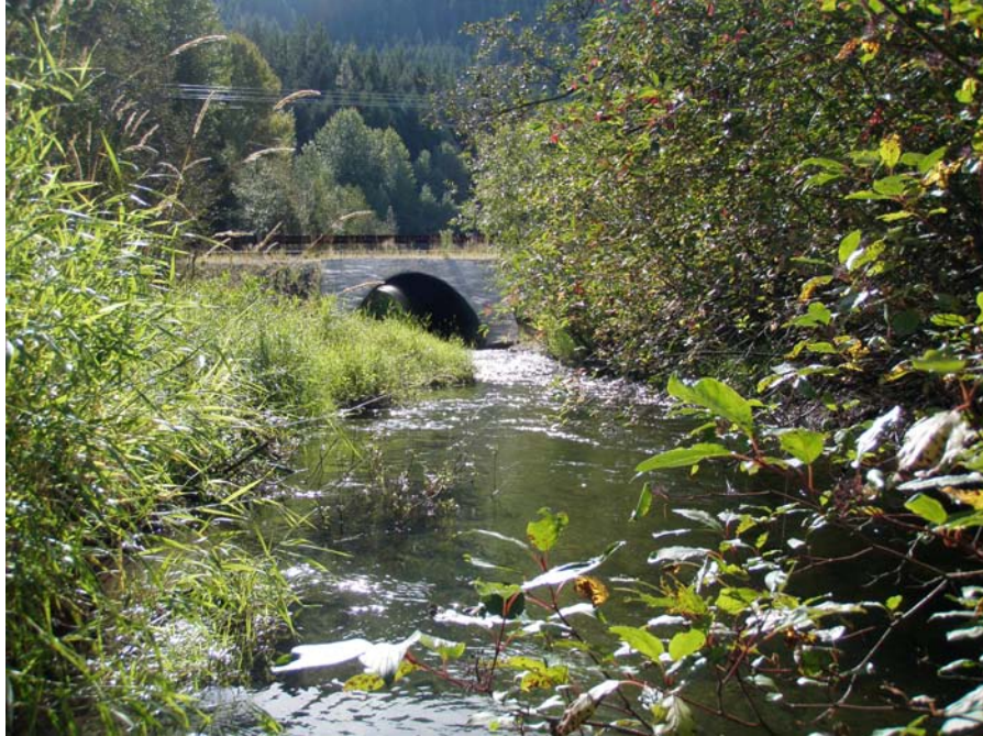
Photograph No. 47. View to the east looking upstream at culvert through improved road embankment that reconnects historic channel path. Lower Nason Creek, Wenatchee Subbasin, Washington – Bureau of Reclamation Photograph by E. Lyon, September 15, 2010.
