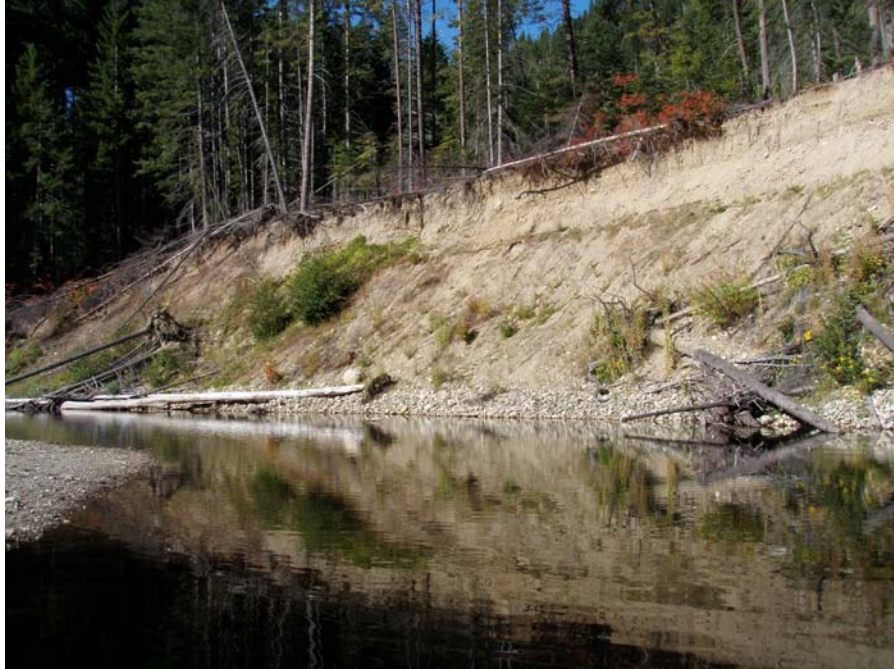
Photograph No. 23. View to the southwest looking upstream at an eroding glacial deposit overlying the Chumstick Formation along river left. Lower Nason Creek, Wenatchee Subbasin, Washington – Bureau of Reclamation Photograph by E. Lyon, September 14, 2010.
