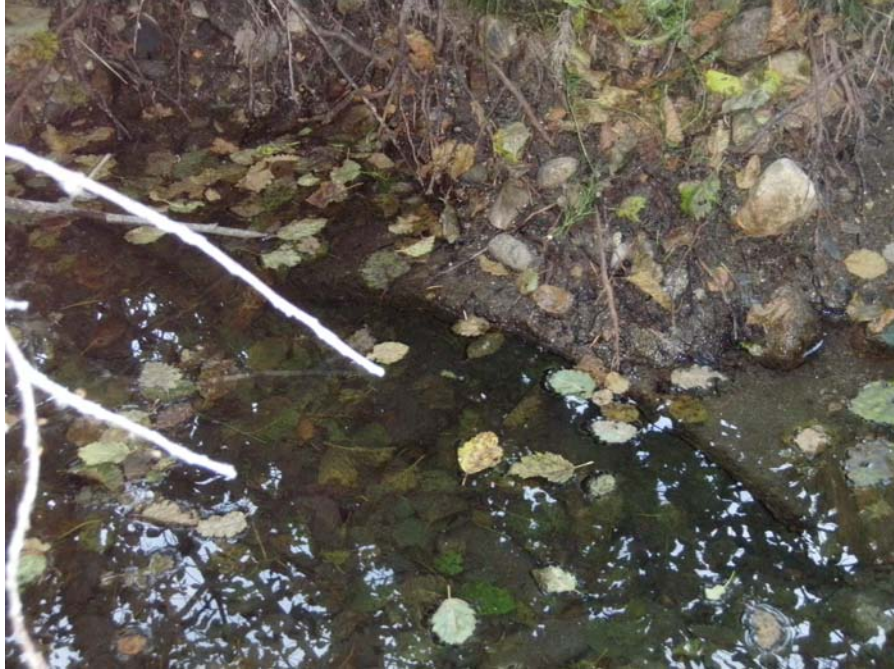
Photograph No. 57. View to the west looking at concrete culvert that poorly connects historic channel path through improved road embankment. Lower Nason Creek, Wenatchee Subbasin, Washington – Bureau of Reclamation Photograph by E. Lyon, September 16, 2010.
