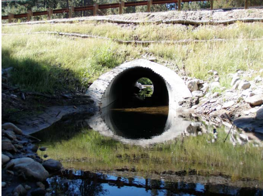
Photograph No. 13. View to the west looking upstream at a culvert placed through improved road embankment to reconnect side channel along river right. Lower Nason Creek, Wenatchee Subbasin, Washington – Bureau of Reclamation Photograph by E. Lyon, September 13, 2010.
