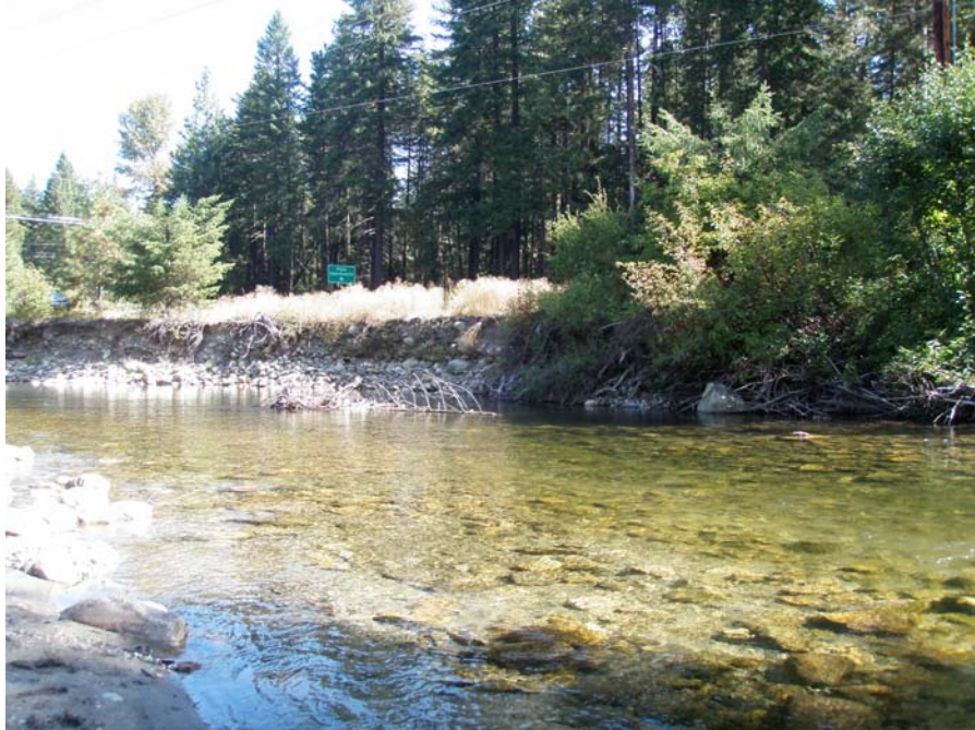
Photograph No. 5. View to the northeast looking at bank erosion along river right that could threaten improved road. Lower Nason Creek, Wenatchee Subbasin, Washington – Bureau of Reclamation Photograph by E. Lyon, September 13, 2010.
