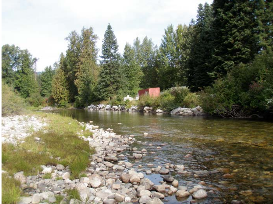
Photograph No. 49. View to the north looking downstream at riprap placed along river right. Lower Nason Creek, Wenatchee Subbasin, Washington – Bureau of Reclamation Photograph by E. Lyon, September 16, 2010.
