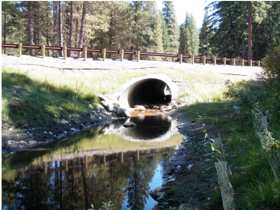
Photograph No. 16. View to the southeast looking upstream at culvert placed through improved road embankment that reconnects side channel. Lower Nason Creek, Wenatchee Subbasin, Washington – Bureau of Reclamation Photograph by E. Lyon, September 13, 2010.
