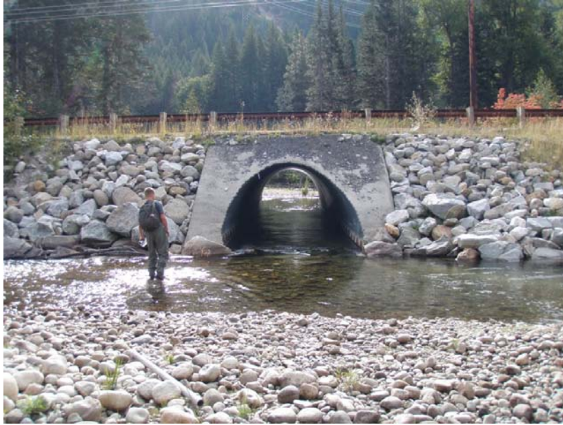
Figure 16. Channel Segment A: View looking at culvert placed through State Route 207 near RM 3.90 that reconnects historic channel path (side channel SC_3.48_R). Lower Nason Creek, Wenatchee Subbasin, Washington – Bureau of Reclamation Photograph by E. Lyon, September 15, 2010.
