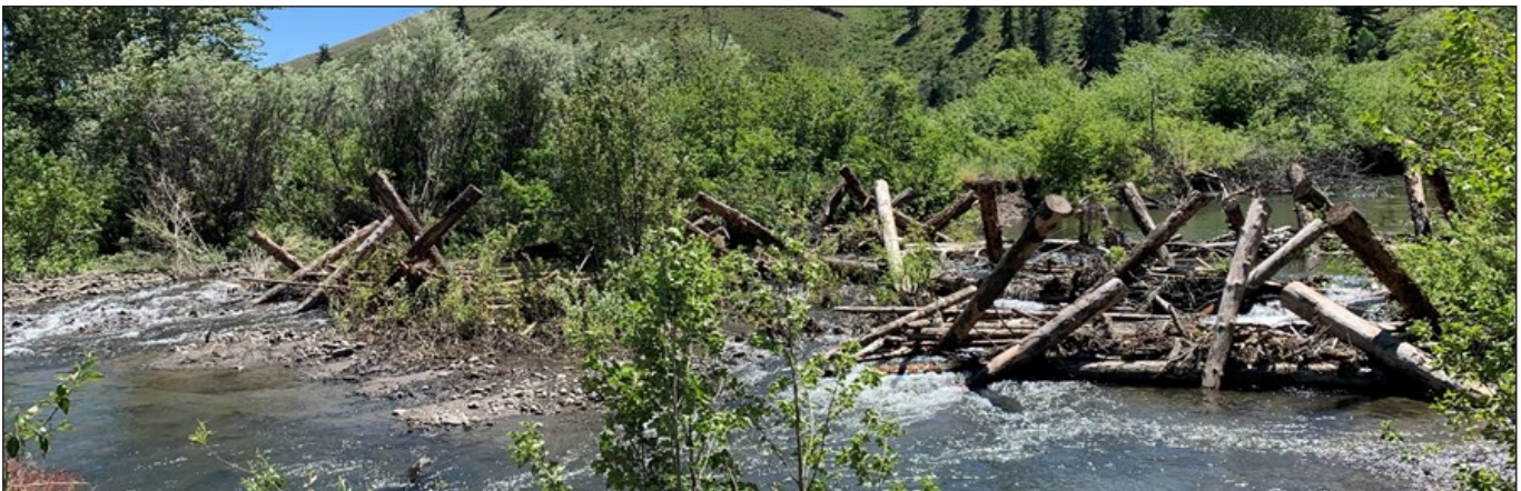
Above: Five engineered log jams and 10 rootwads were placed in the Ragland Reach for habitat enhancement.
