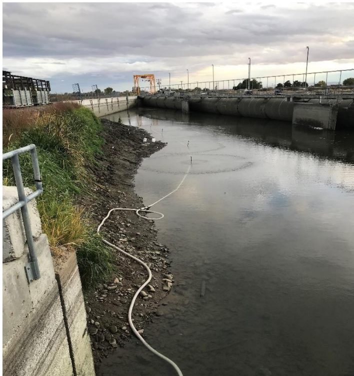
Figure 8. Overview of the PVC sprinkler system deployed upstream of the fish screens in the Wapato Canal in October 2019 immediately after dewatering. The sprinkler spray was directed towards the wetted area in anticipation that the water level would drop overnight, exposing additional sediment and lampreys. The same system was deployed in 2020 as well.
