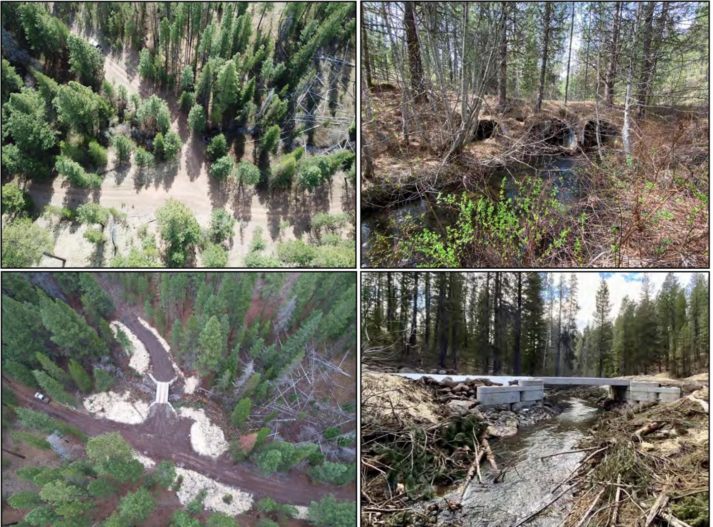
Before (top row) and after conditions following the replacement of an undersized culvert associated with the 191 Road in the White Creek watershed. (YN)
