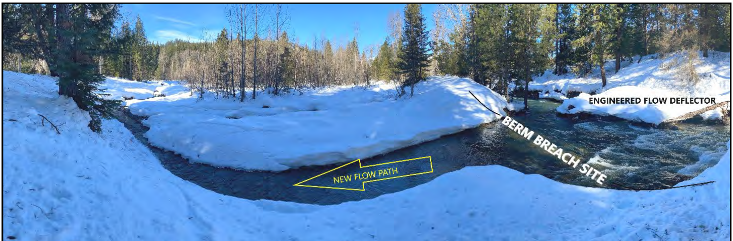
River mile 5.86 where a berm was breached and an engineered flow deflector was installed creating a new floodplain flow path. (YN)
