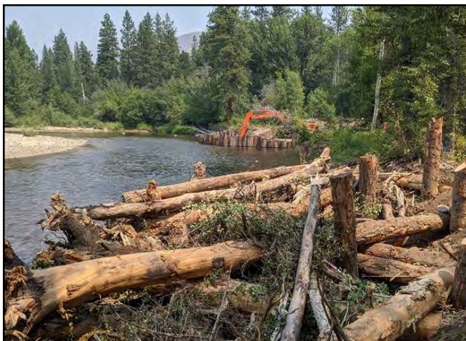
Large wood structure installed in the main channel of the Chewuch River. (YN)
