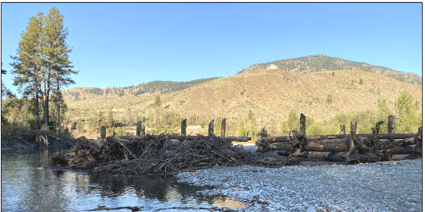
Floodplain roughness (top), bar-apex (middle), and split-flow (lower) log structures were installed in the Methow River to recover natural processes that create and sustain productive fish habitat. (YN)
