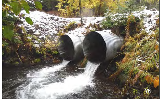
Above: Pre-project conditions, illustrating fish passage issues.
