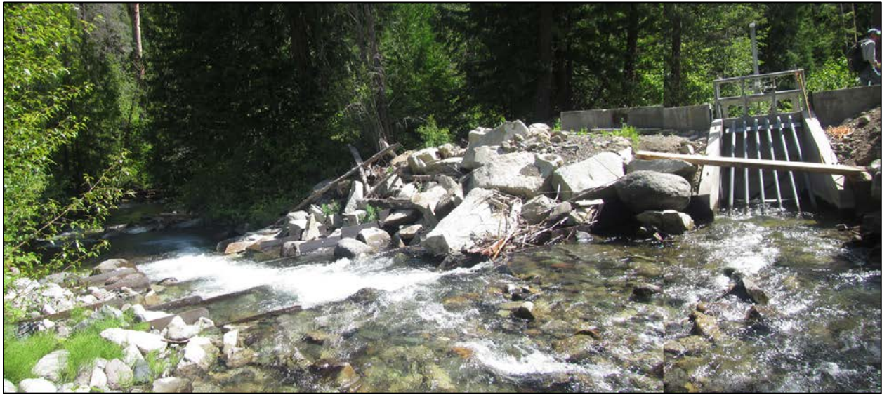
Figure 77. Wolf Creek diversion gate and downstream constructed steel plate weirs at RM 4.53. (Photo: 7/8/2020)
