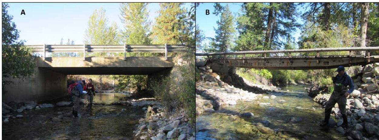
Figure 38. A) Wolf Creek Road (RM 0.03) crossing and related large boulder weirs at and upstream. B) Railroad car bridge with cement footings and large boulder riprap and raised access road prism. (Photos: 10/1/2019)
