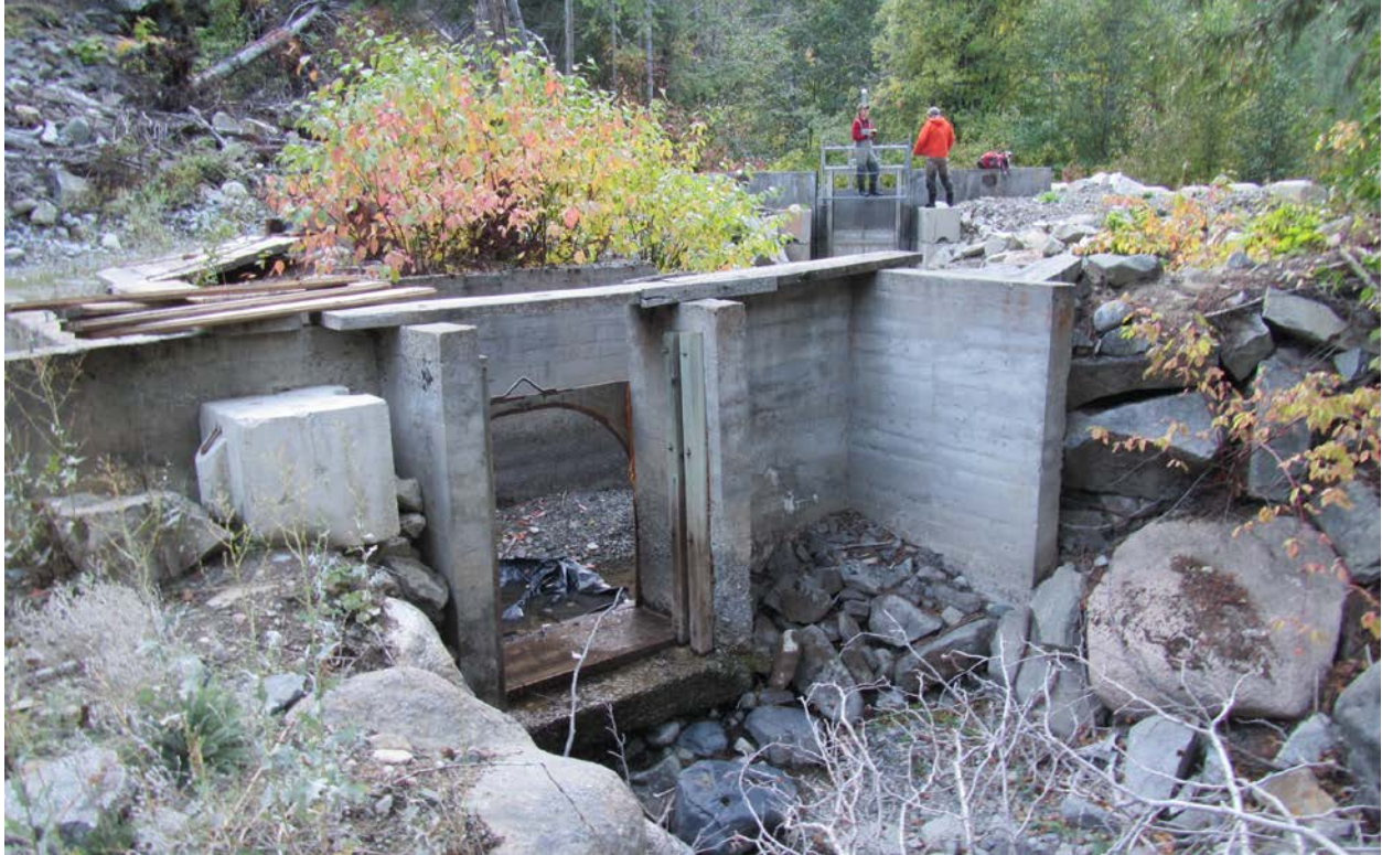
Figure 11. Wolf Creek diversion withdrawal gate, ditch, and overflow return gate (foreground). (Photo: 10/5/2019)
