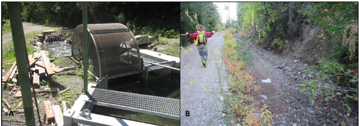
Figure 78. A) Fish screen that leads into Wolf Creek irrigation ditch buried under access road (Photo: 7/8/2020) B) Wolf Creek irrigation open ditch down valley along access road (Photo: 10/5/2019)
