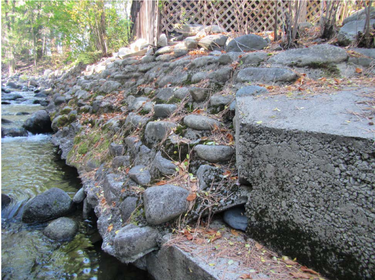
Figure 8. Cement bank armoring and upstream levee on river left near a home in Reach 1 with undercut erosion occurring. (Photo: 10/1/2019)
