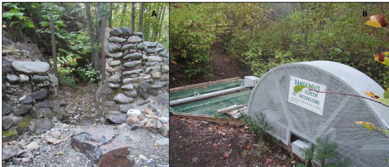
Figure 49. A) irrigation outtake at RM 1.44; B) fish screen associated with irrigation outtake and ditch.
