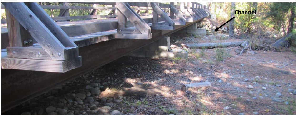
Figure 34. Private bridge crossing at RM 0.3. Photo at downstream side of bridge on river right looking across active channel where sediment is accumulating. Low-flow channel in background next to boulder gabion and riprap. (Photo: 10/1/2019)
