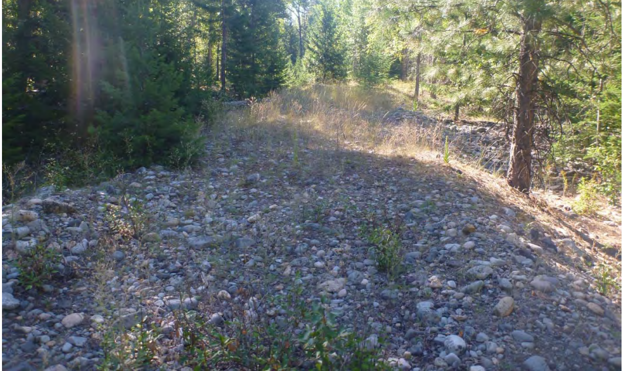
Figure 93. Section of the breached push-up levee on the floodplain near RM 71.1. (8/26/2014)
