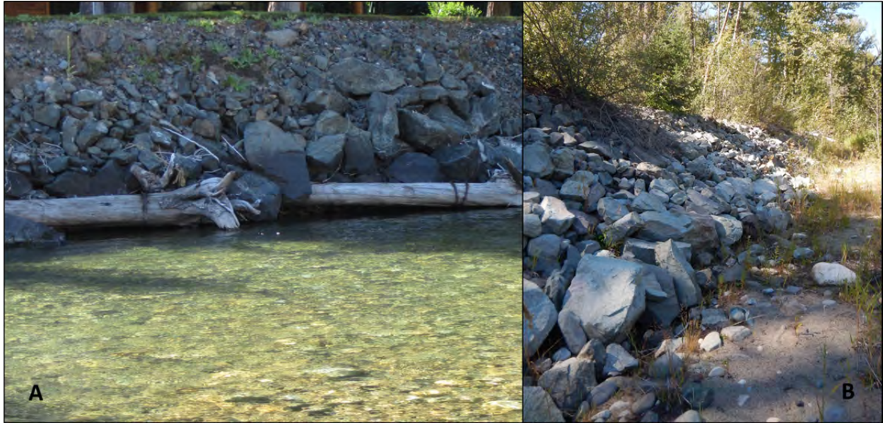
Figure 46. Examples of confining features constructed of large angular riprap in Reach 2, (A) riprapped bank with cabled and anchored logs on river-right at RM 62.7; (B) section of the levee composed of riprap on river-right at RM 63.5. (9/4/2014)
