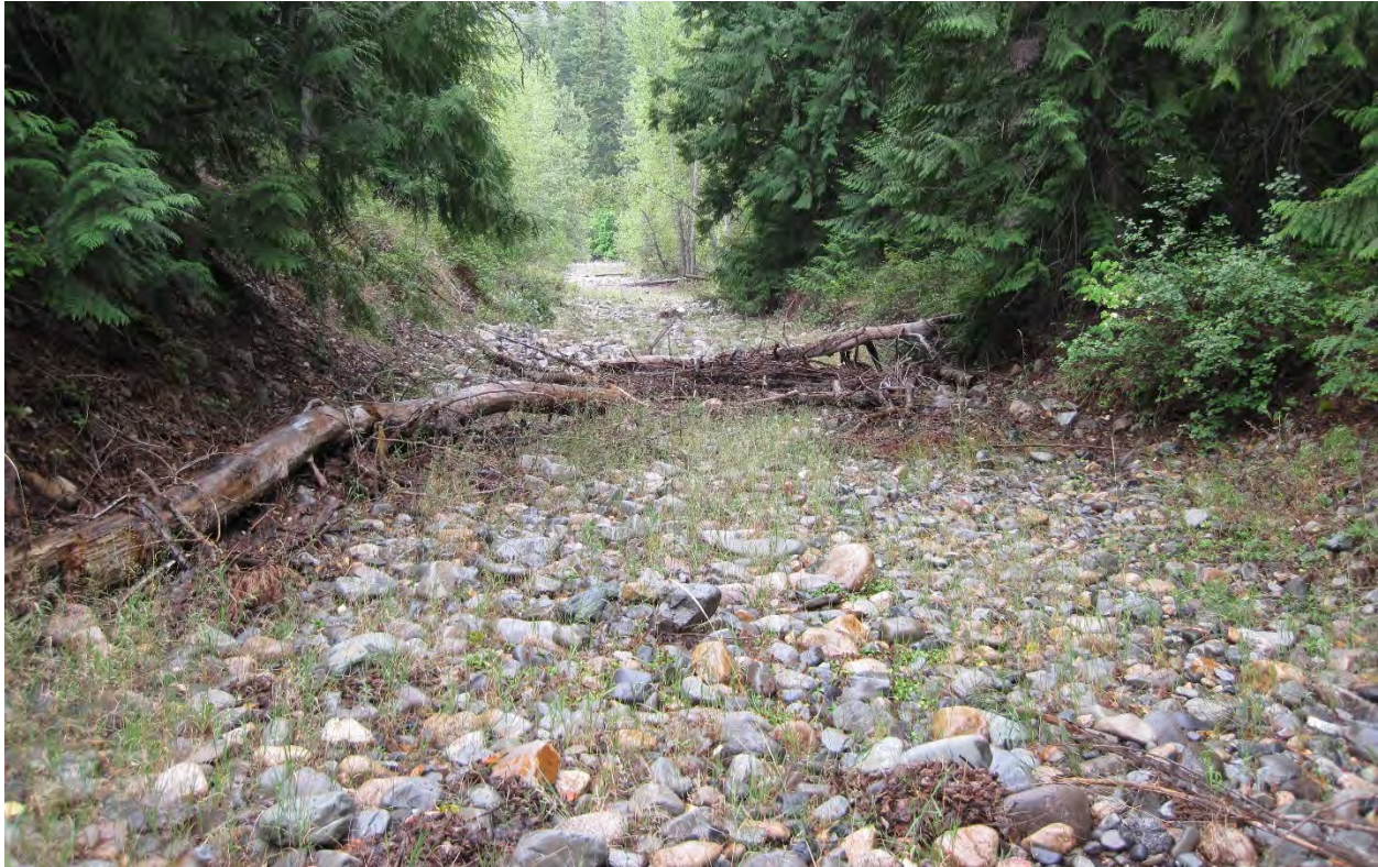
Figure 108. Constructed canal that drains surface water from the floodplain and disconnects a side-channel. Photo taken at the downstream end looking up-canal near RM 73.45. (8/14/2014)
