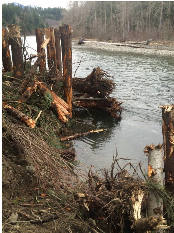
Figure 11 Completed Type 1 engineered log jam. Care was taken to ensure the structures did not produce a “straining” effect to improve boater safety.
