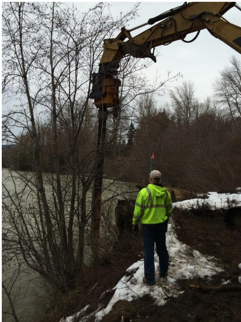
Figure 6 Habitat conditions during pile driving activities with a Movax. Note: flows were elevated and water was naturally turbid at the beginning of the project construction activities
