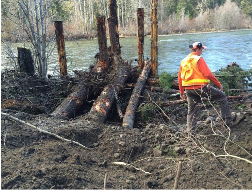
Figure 12 Furthest downstream engineered log jam near completion. This site proved challenging in that the total specified piles were not able to be driven to specified depth. A new design was engineered to mitigate the lack of piles which included increased bank excavation, installation of whole, small diameter trees in the back water downstream of this image. Two ELJ's worth of materials were installed at this one location. The end result more than doubled juvenile salmonid rearing and forage habitat.
