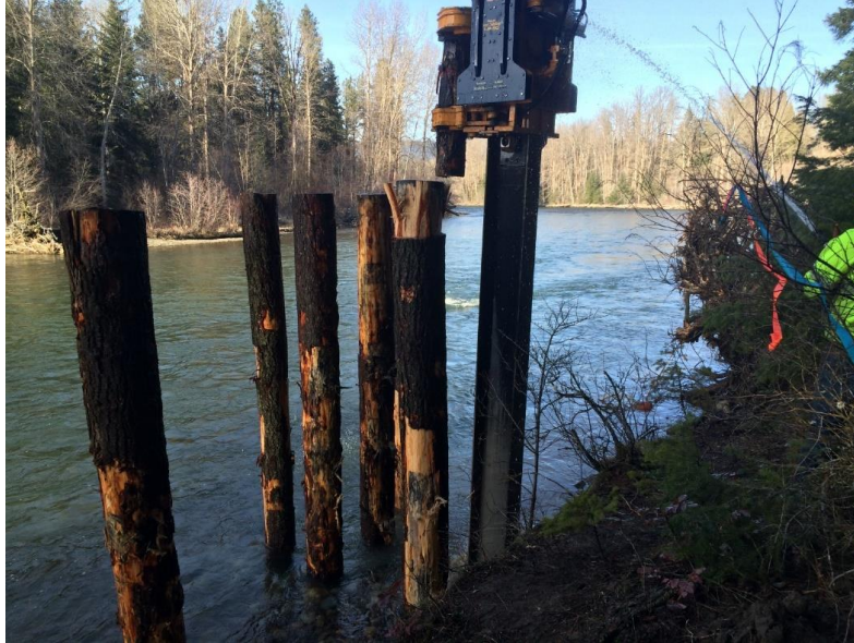
Figure 9 Habitat conditions during pile driving activities. An H-pile was used which essentially pre-drilled the bore to speed efficiency of pile driving and ensure all piles were driven to depth.
