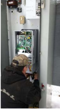
Figure 1. Mark Luce of Laurmar Electric installing variable speed drive in well #1. Variable speed drive is a more efficient way of operating wells for the Cle Elum Facility.
