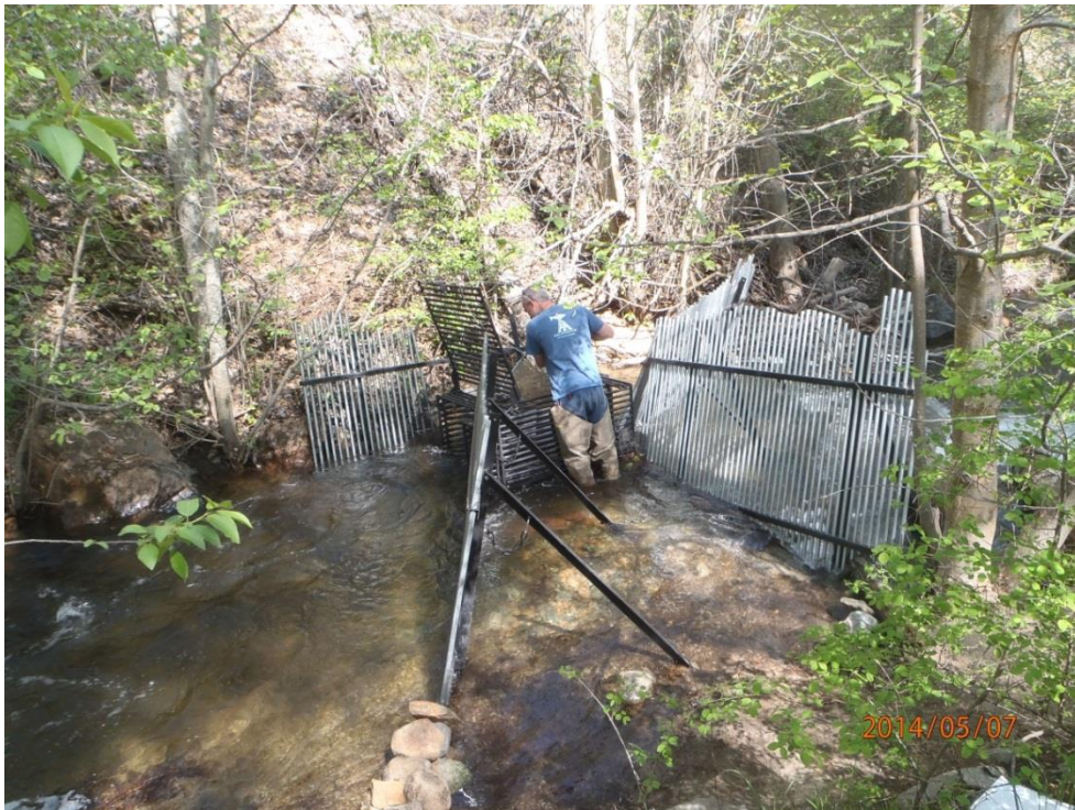
Figure 2.4 - South Fork Gold Creek weir
