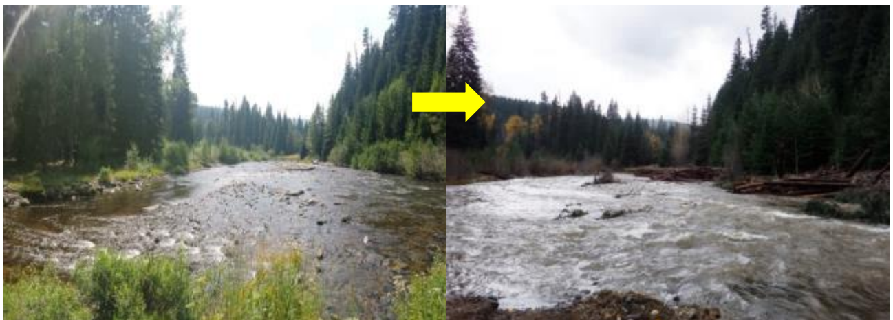
Figure 7. Pre- (left) and post-project (right) photos of constructed log jams along the right bank of the Klickitat River adjacent to 255 road.
