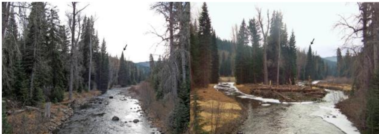
Figure 5. Pre- (left) and post-project (right) photos looking downstream from the 255 road crossing of the Klickitat River.
