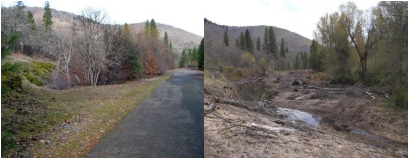
Figure 11. Klickitat River Floodplain Conservation and Restoration– Phase 3 pre (left) and after (right) removal of road prism, construction of channel and grading of floodplain.
