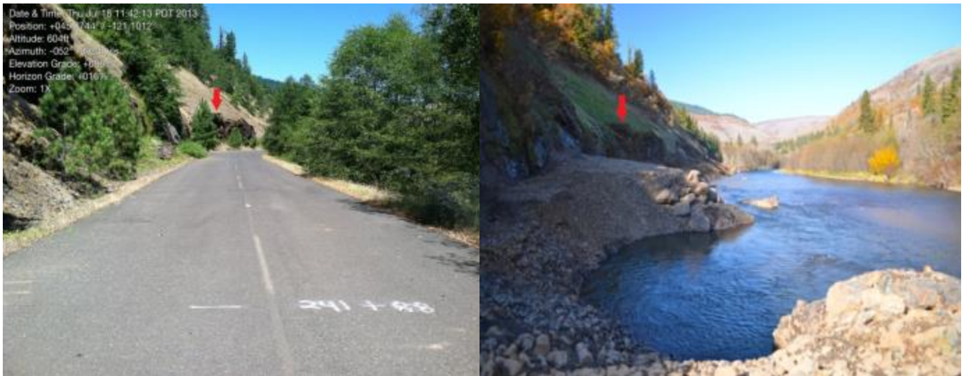
Figure 12. Klickitat River Floodplain Conservation and Restoration– Phase 4 pre (left) and after (right) removal of road prism and exposure of bedrock outcrop.
