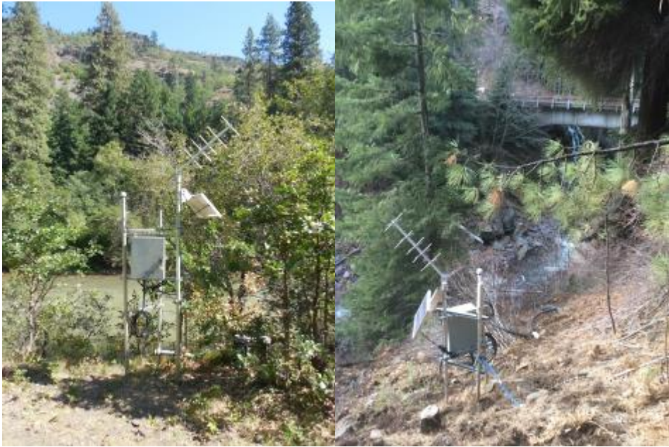
Figure 20. Telemetry communication equipment, Klickitat River DS of Summit Ck (upper left) and Big Muddy Ck @ 255 rd x-ing (upper right).
