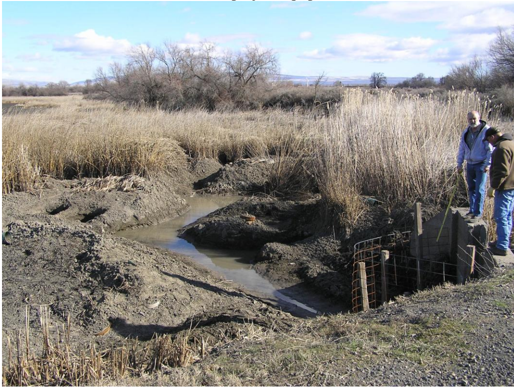
This is the lower end of Bridgeman Pond, where the culvert crosses under McGee Road, and into Morgan Lake. Beaver activity was high, in spite of passive flow.
