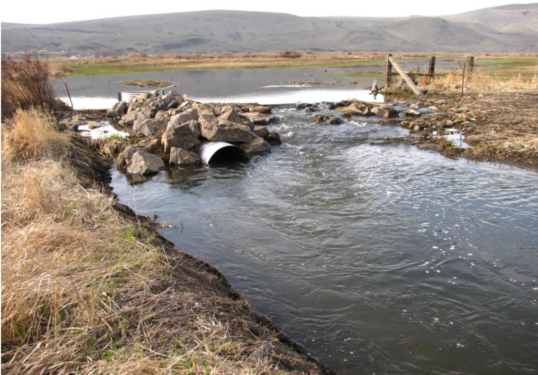
Control Structures operating at high water to pass fish
