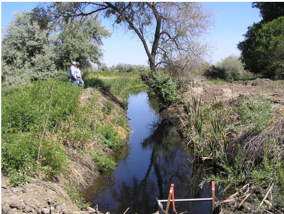
This historic delivery ditch, leading from Morgan Lake, was cleaned to its original elevation and a new water control structure was installed (foreground)
