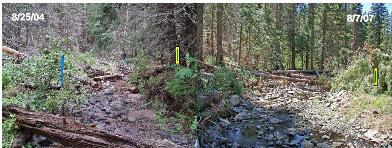
Figure 5. Upstream end of grade control riffle (Station 2+20) before (left) and after (right) construction.
