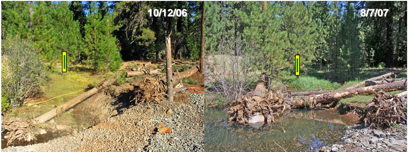
Figure 14. In-progress (10/12/06) and after (8/7/07) photos of Station 20+50 of Tepee Creek IXL Meadows project. Note emergent wetland (behind LWD) created by backwatering and water table rise.
