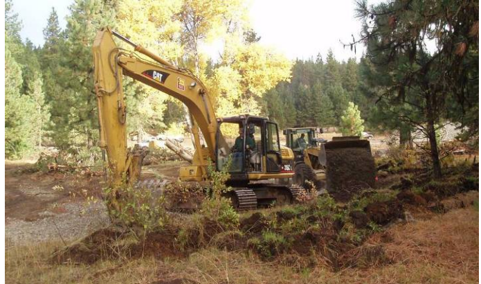
Figure 9. Salvage of sod mats and shrubs (foreground) and gravel fill for riffles (background)
