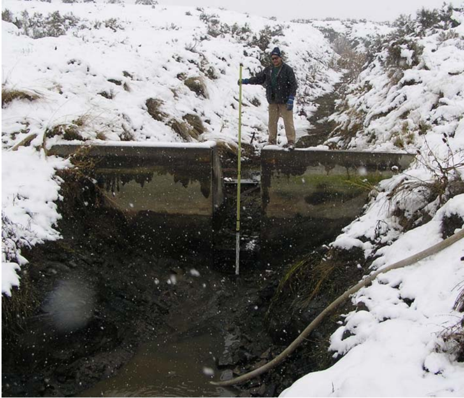
Byron head works at full drawdown and before installation of new control gate
