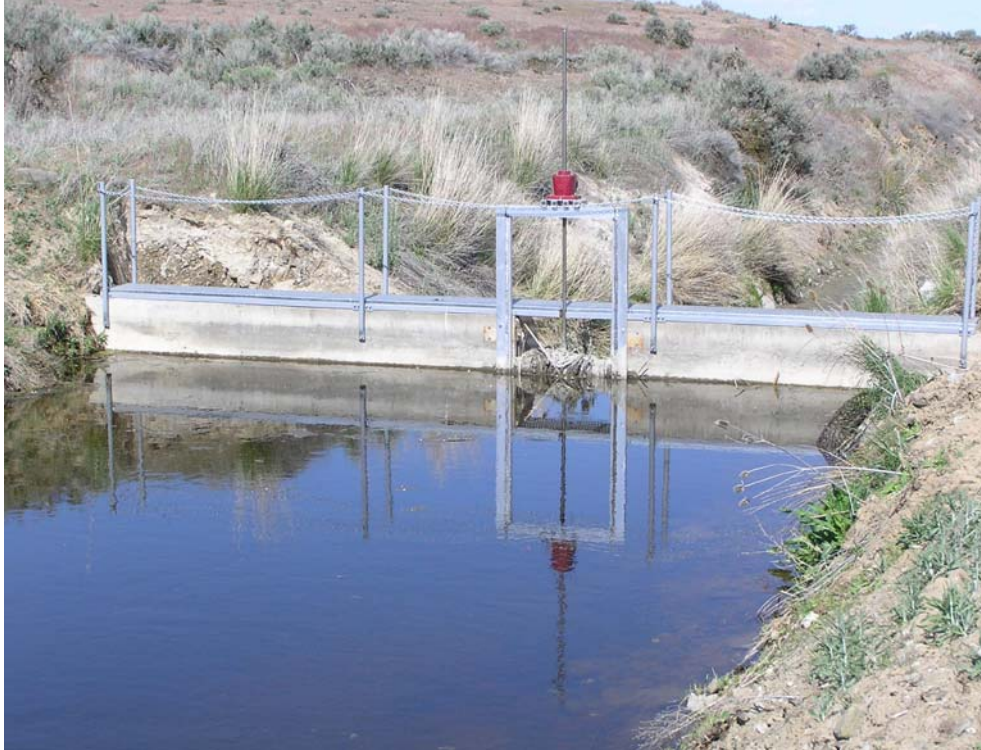
New control gate at nearly full pool
