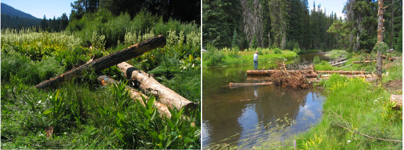
Figure 20. Roughness elements placed at Site C1 along avulsion path (left). In-channel LWD jam constructed at site K5.
