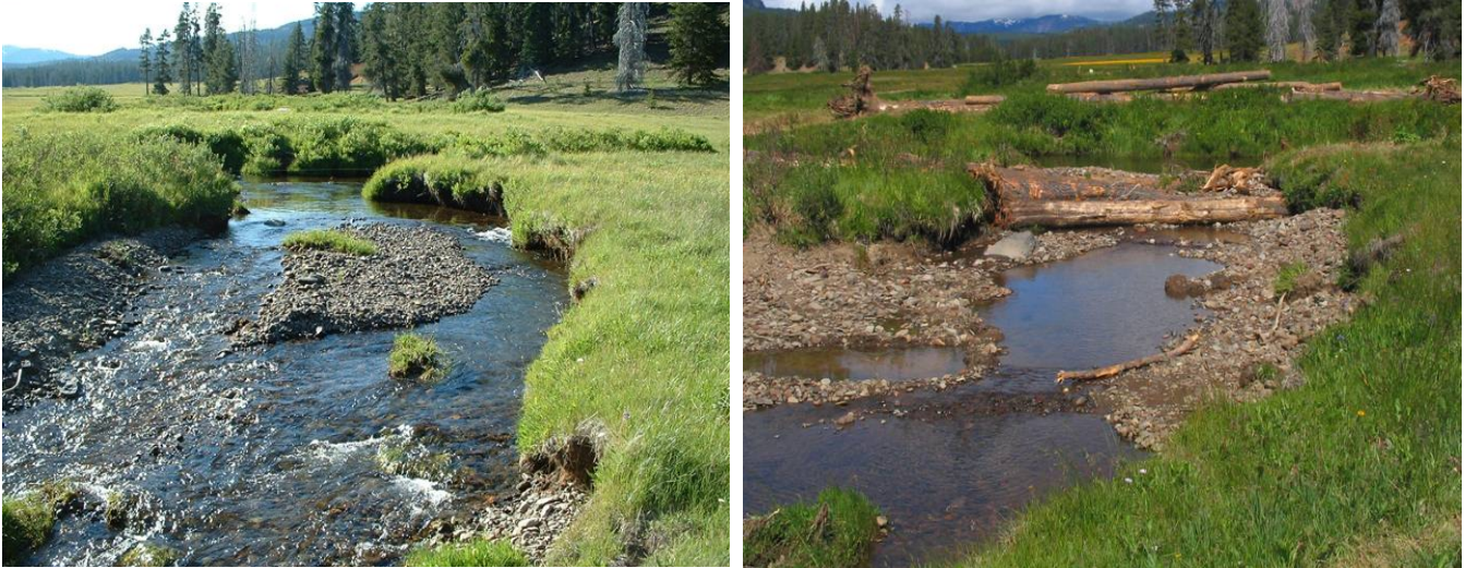
Figure 13. Upstream control for avulsion channel (Site 4, Element 5) before (7/8/03, left) and after construction (7/7/04, right).
