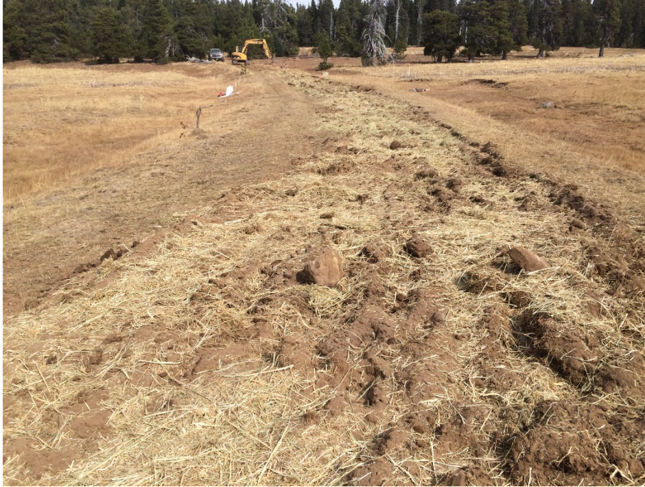
Figure 5 Ripped road resseeded.
