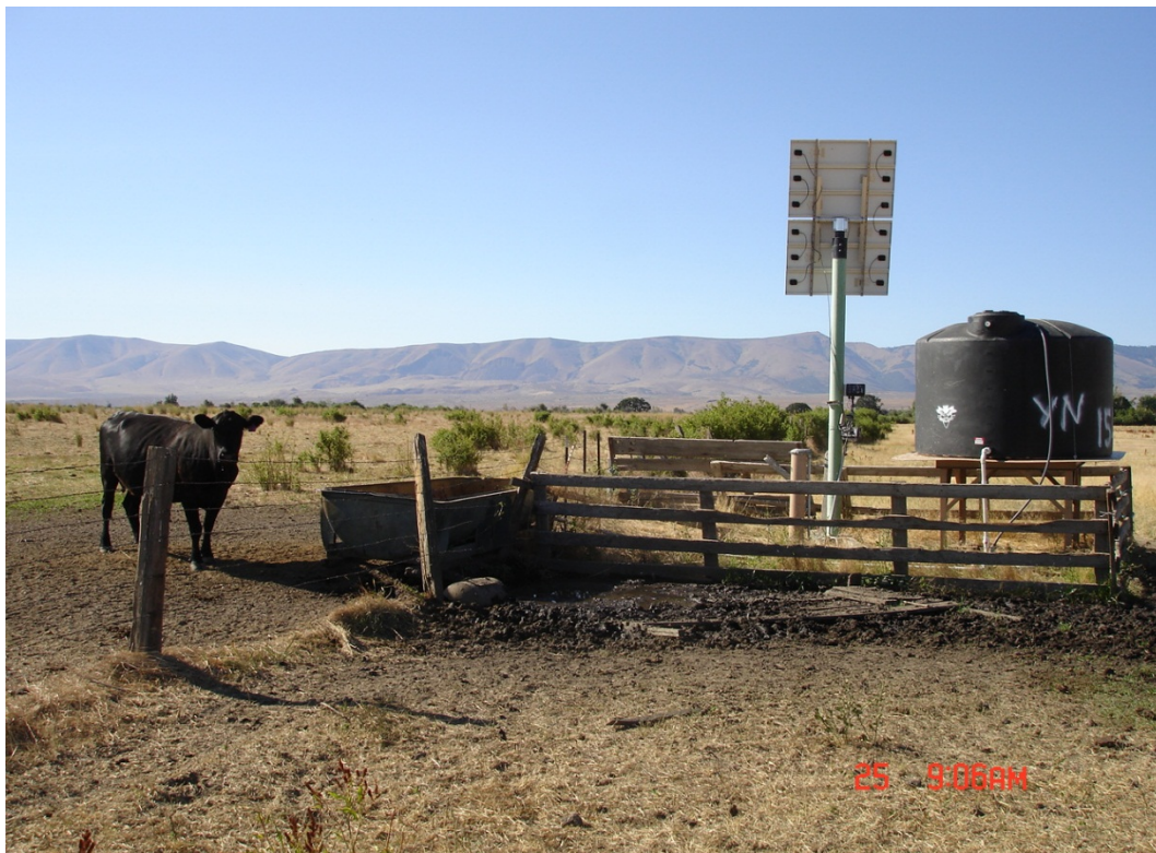
Figure 10. Stock pump and watering trough.
