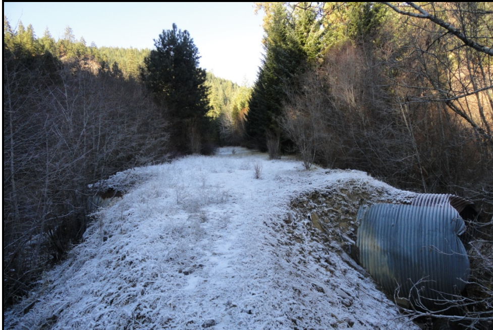
Figure 1. Upstream culvert and road that was later removed. Historic floodplain is to the right of the image and NF Toppenish Creek is to the left.
