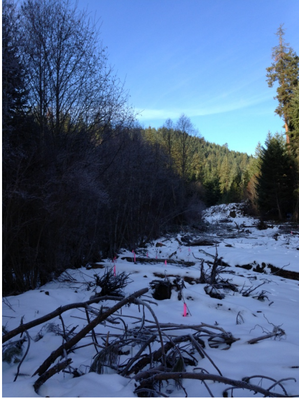
Figure 7. Former road alignment at upper culvert. This photo is the same location as figure 1, post construction.
