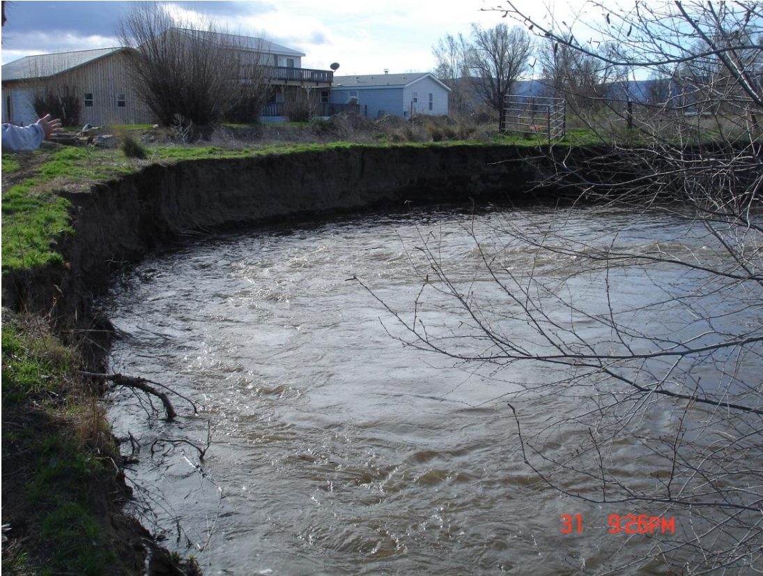
Figure 1. Looking upstream at eroding bank, March 2012
