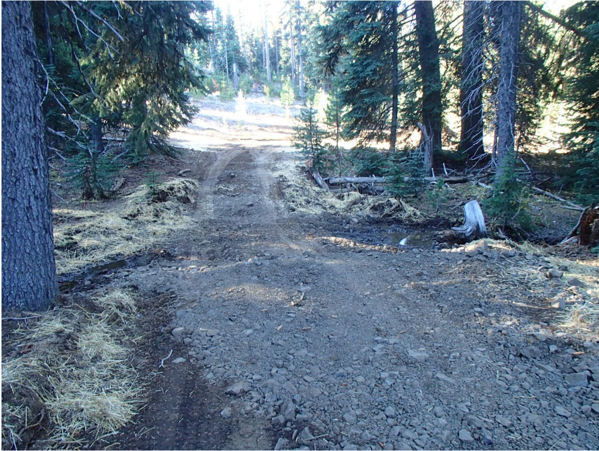
Figure 6. Site condition immediately following construction and revegetation efforts (flow is now perennial through the ford).
