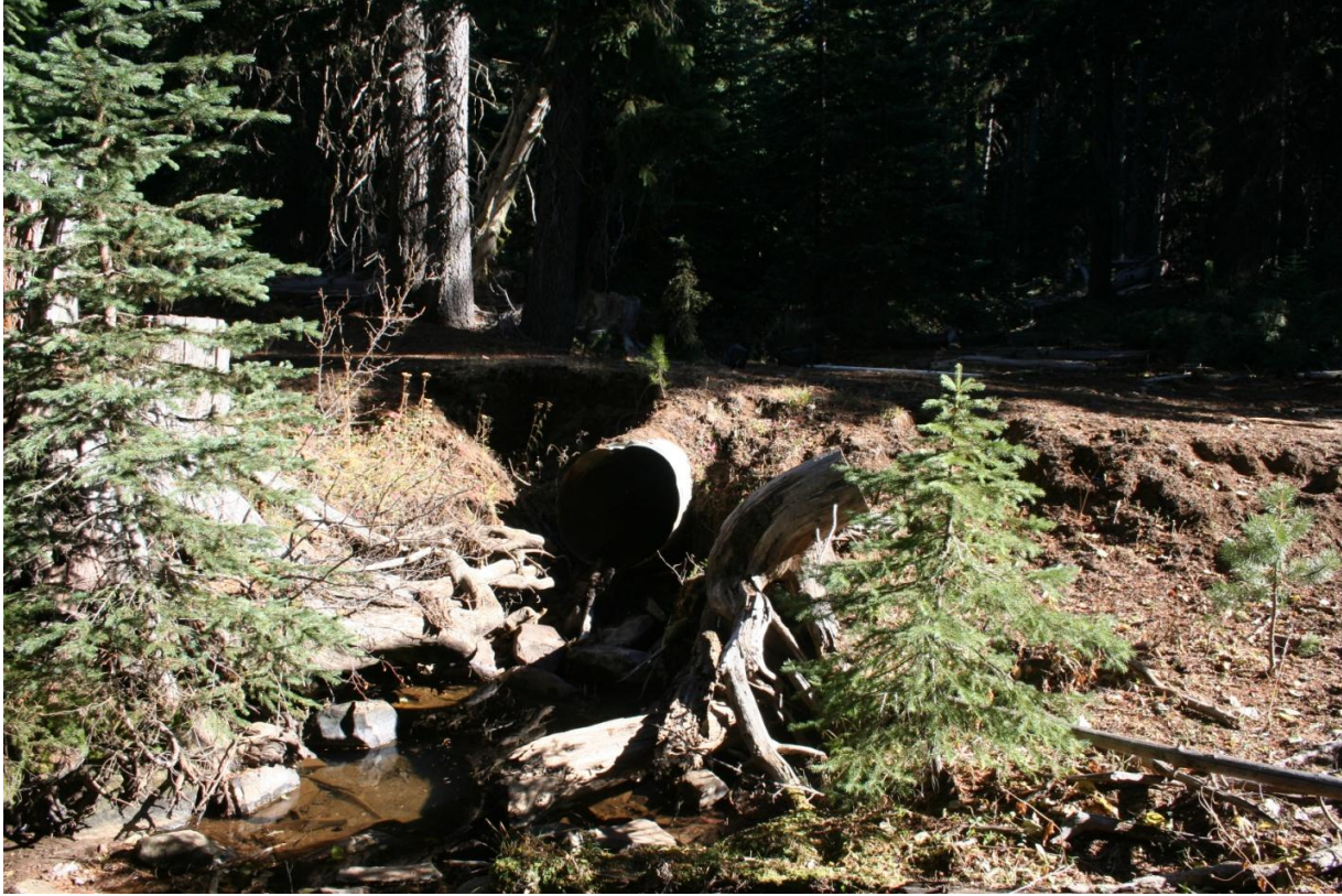
Figure 3. Inoperable culvert at channel crossing prior to implementation. Note: 2' drop at culvert outlet
