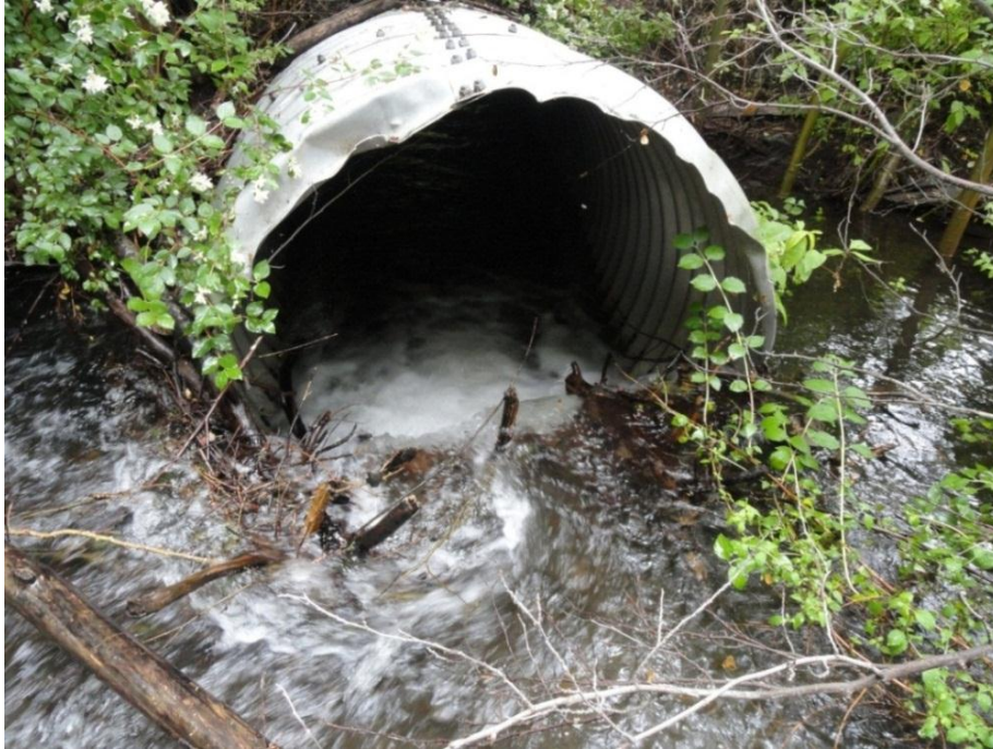
Figure 14. Clogged culvert causing creek to partially reroute
