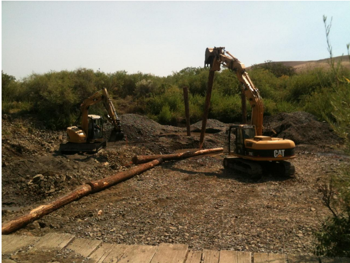
Figure 3. Roughened channel complete upstream to the dam. Excavator to the right is ~14' higher in elevation than the elevation of the pre treatment channel elevation condition. The excavator to the left is positioned where the woody berm was constructed.
