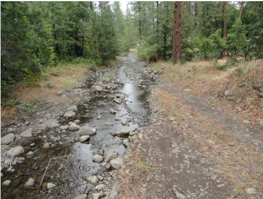
Figure 15. Creek re-routed down the road due to clogged culvert.
