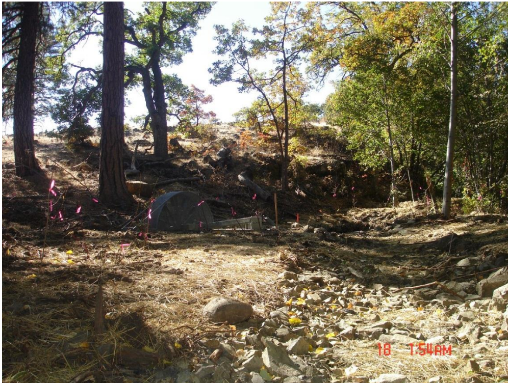
Figure 12. Photo illustrating fish screen and overflow channel. Impacted area was seeded and mulched. Pink flags indicate planted container plants.
