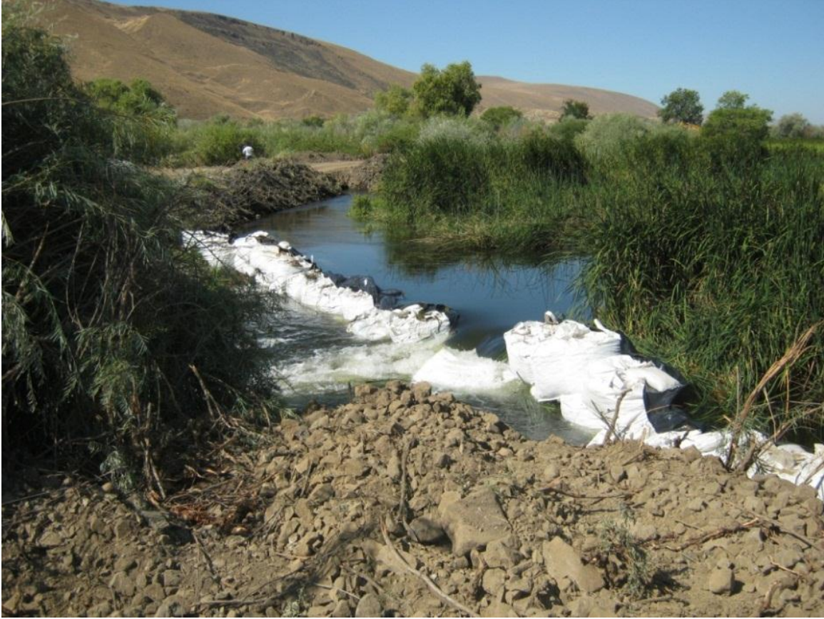
Figure 31. Failed coffer dam attempt using bulk bags.
