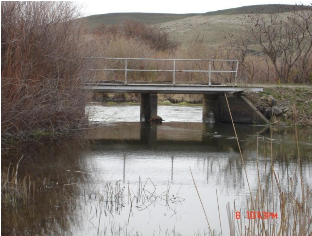
Figure 29. Obsolete Irrigation Diversion (Durham Dam) located on Toppenish Creek.
