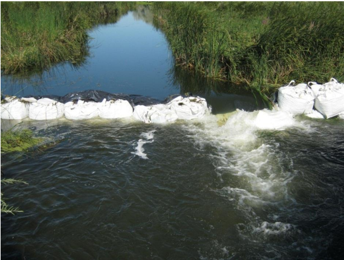
Figure 30. Failed coffer dam attempt using bulk bags.
