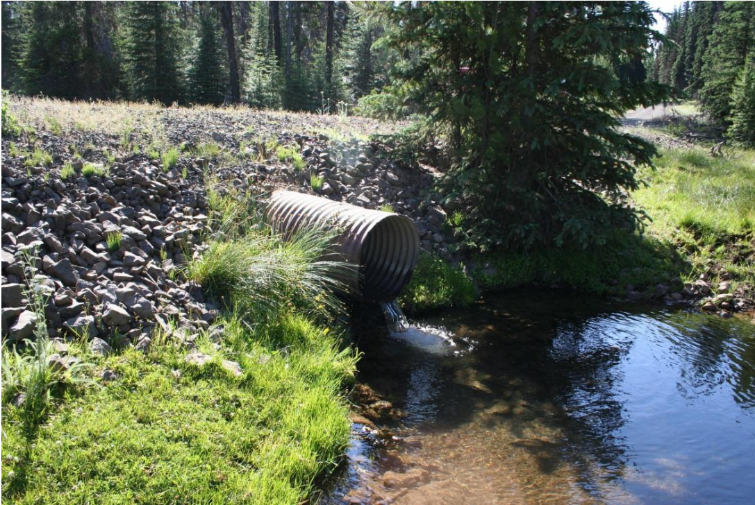
Figure 24. Culvert # 1. Outfall of the culvert on the Rd. 80 crossing of Panther Creek
