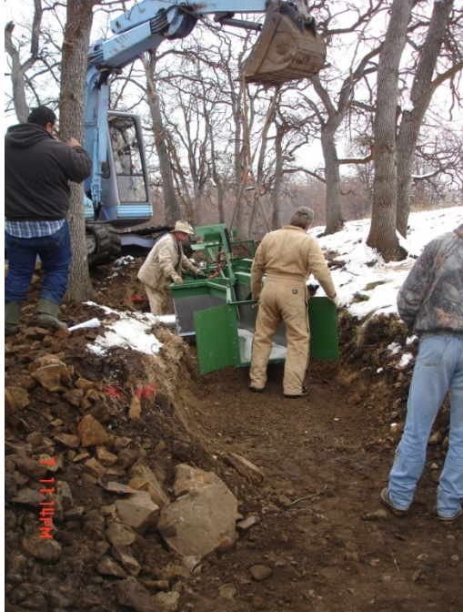
Figure 14. Winter of 2010 4 CFS Rotary Wiper W/ Guard fish Screen installed.
