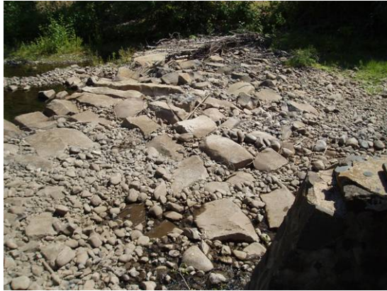
Figure 1. Photo of the Olney- Lateral Diversion in the drought year of 2005 creating a passage barrier
