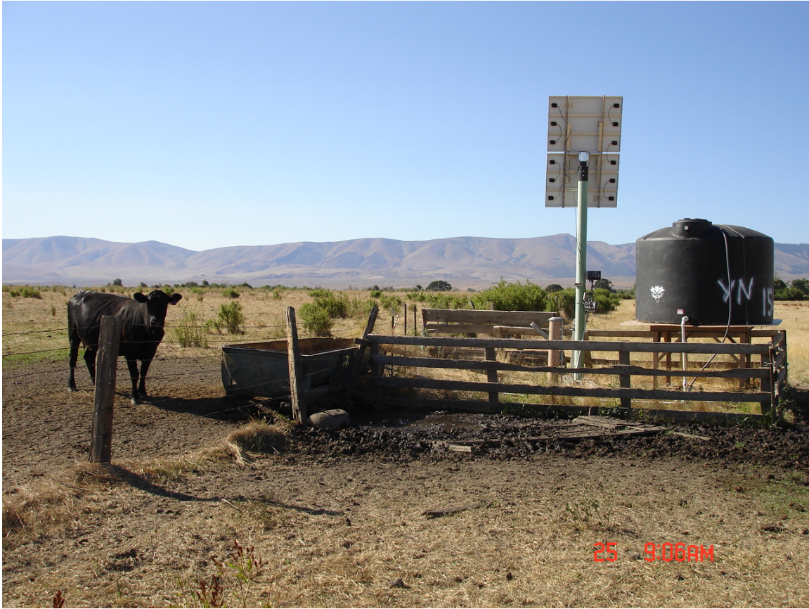
Figure 26. Stock pump and watering trough.
