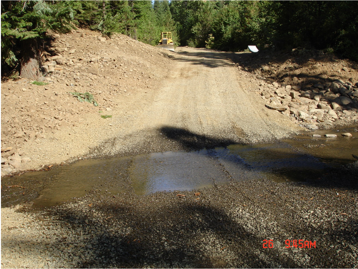
Figure 11. New armored crossing topped with 5/8 minus crushed gravel. Armor rocks are seen on the right.
