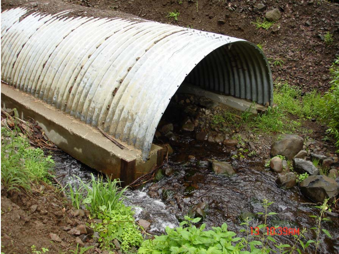
Figure 8. Upper culvert with exposed footings
