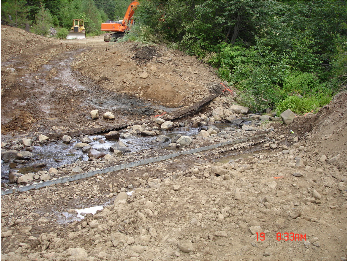
Figure 12. Spring that had been hidden by culvert fill (top left of photo)
