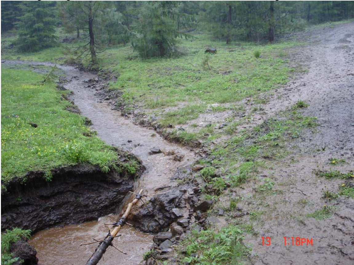
Figure 8. Headcut, SF Simcoe Creek Tributary, prior to road obliteration and stabilization.
